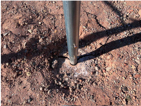
PHOTO 4: Cracked concrete in base of post after dual post test
