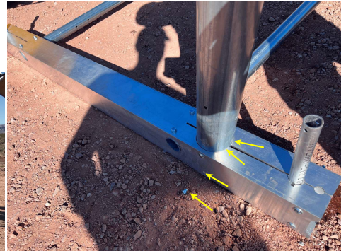
PHOTO 3: Sheared bolt and minor aluminum tube deformation
