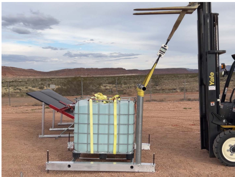
PHOTO 4: 3 rd test with additional ground spikes installed at the back end of the frame.
