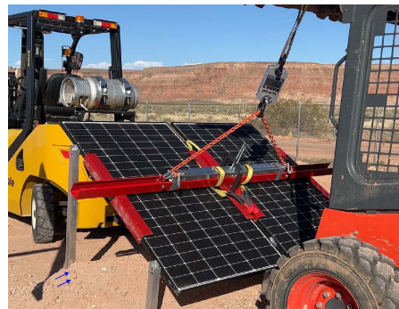
PHOTO 5: Test 1 - Evidence of ballast shift
