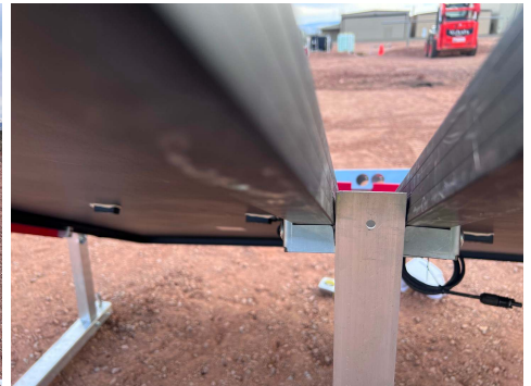
PHOTO 12: Middle brackets after testing
