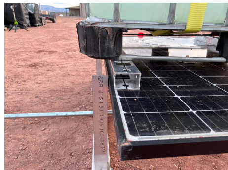
PHOTO 8: Slight deflection noted under load
