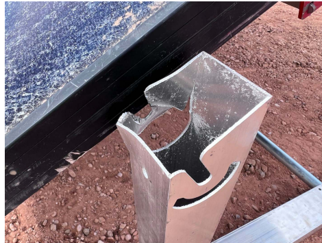
PHOTO 14: Upright mount deformation after testing
