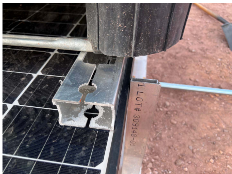
PHOTO 7: Slight deflections noted under load
