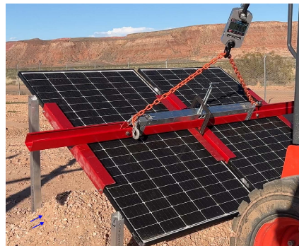
PHOTO 8: Test 2 - Evidence of ballast shift
