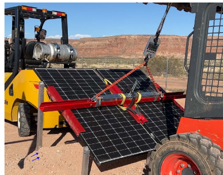
PHOTO 5: Test 1 - Evidence of ballast shift
