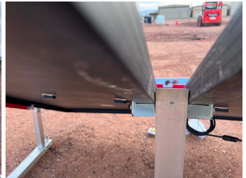
PHOTO 12: Middle brackets after testing
