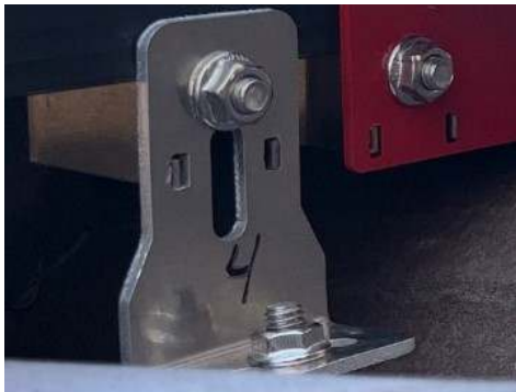
PHOTO 5: Bracket under load
