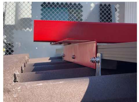
PHOTO 3: Brackets with no load
