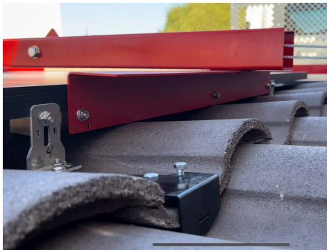
PHOTO 2: Bracket with no load
