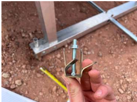
PHOTO 13: Bracket deformation after testing
