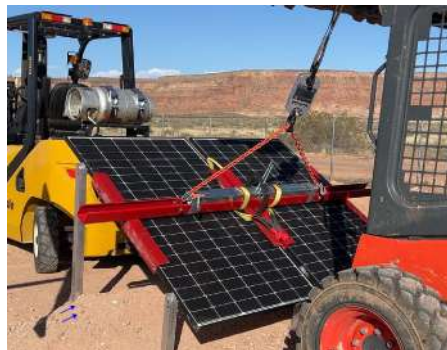
PHOTO 5: Test 1 - Evidence of ballast shift
