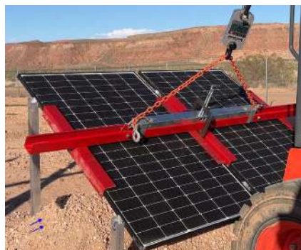
PHOTO 8: Test 2 - Evidence of ballast shift
