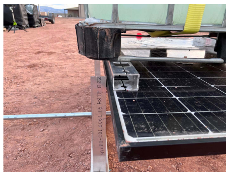
PHOTO 8: Slight deflection noted under load
