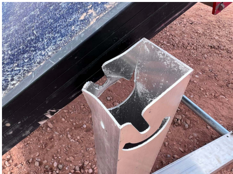
PHOTO 14: Upright mount deformation after testing
