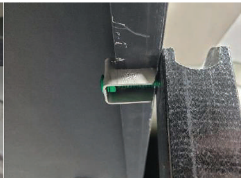
Figure 18: IR Ballast frame connection to solar panel
