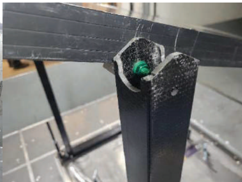
Figure 17: IR Ballast frame connection to solar panel
