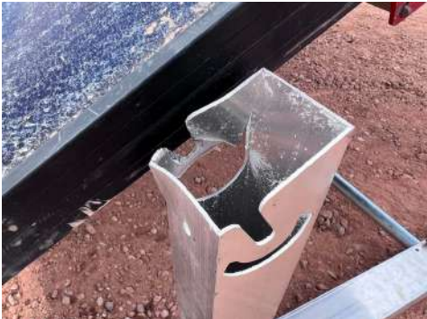
PHOTO 14: Upright mount deformation after testing
