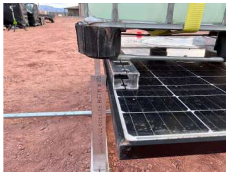
PHOTO 8: Slight deflection noted under load
