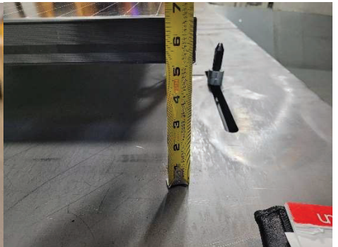
Figure 6: Height from roof to panel, Runs 2 & 3
