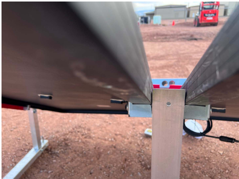
PHOTO 12: Middle brackets after testing
