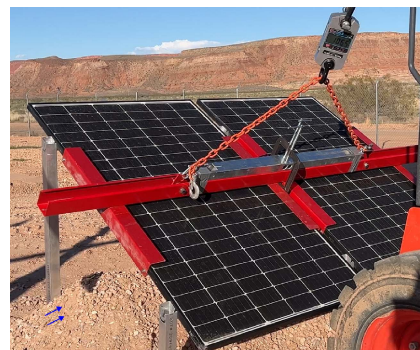
PHOTO 8: Test 2 - Evidence of ballast shift
