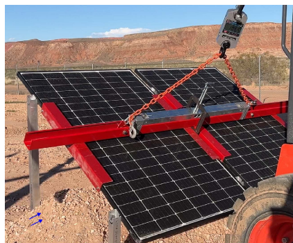
PHOTO 8: Test 2 - Evidence of ballast shift
