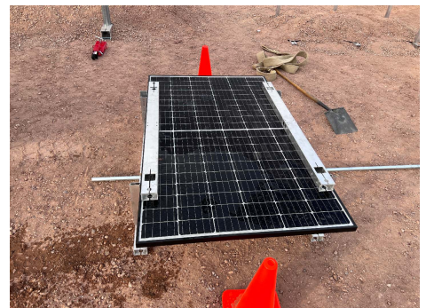
PHOTO 9: IR-30 system after compressive load tests
