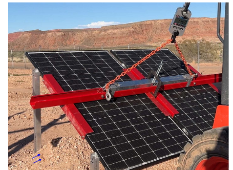
PHOTO 9: Test 2 - Evidence of ballast shift
