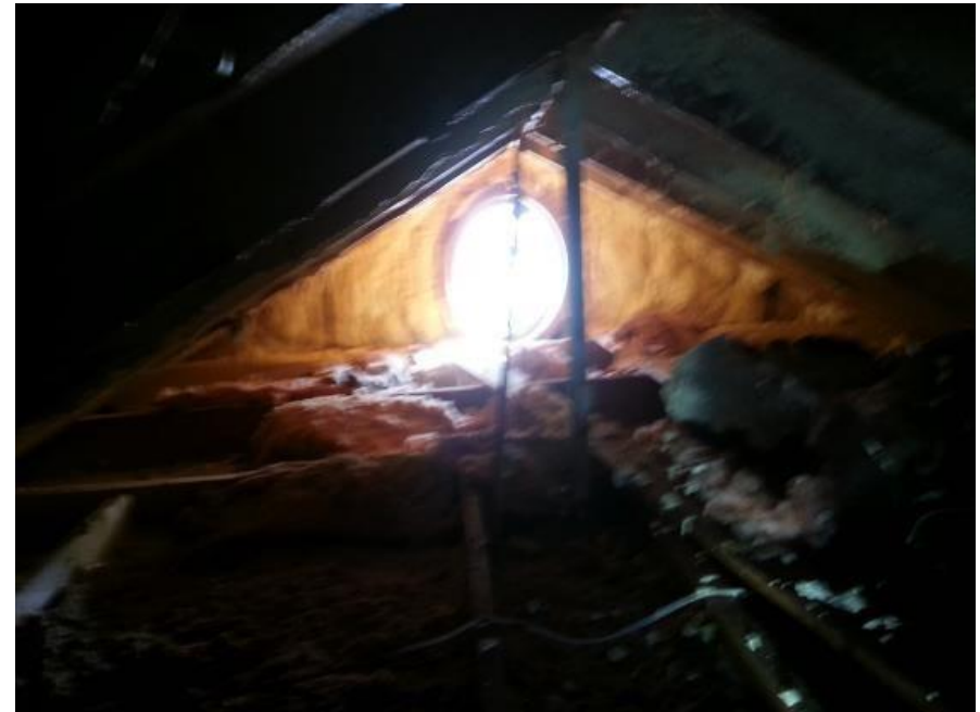
Window not sealed
