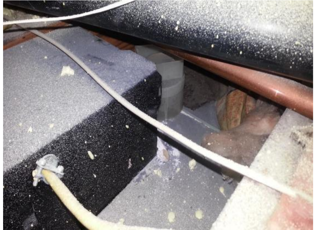
Bathroom vent to attic
