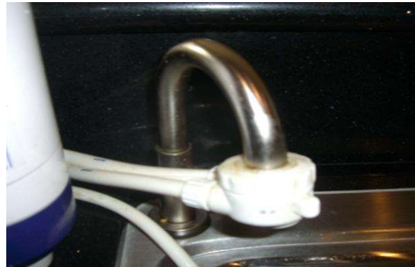
Second-installed faucet onto the same sink
