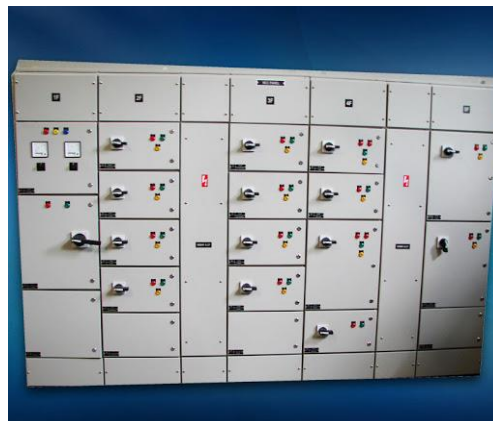
VFD Panel and MCC panel
