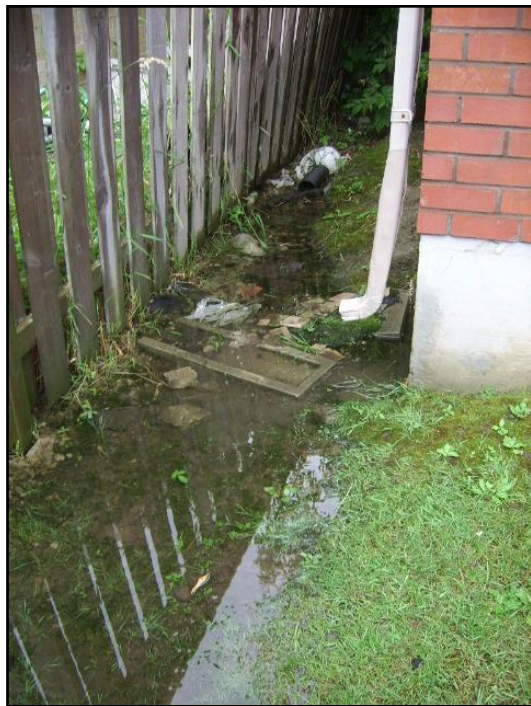
Downspouts end too close to building
