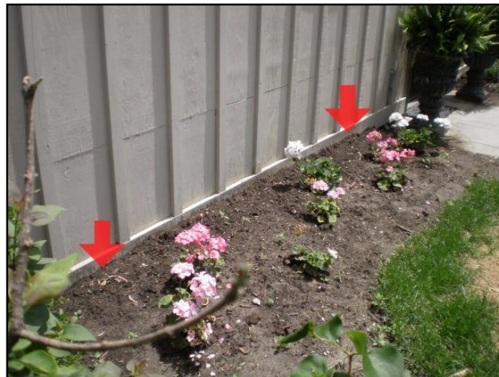
Too close to grade
