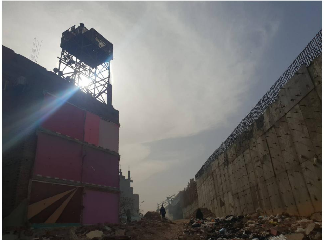
Khairallah district during the widening of the ring road construction mobie photos, taken by Azza Ezzat, 2022
