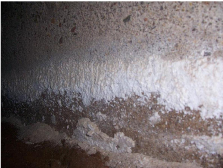
Figure 1. Excessive efflorescence on foundation wall.
