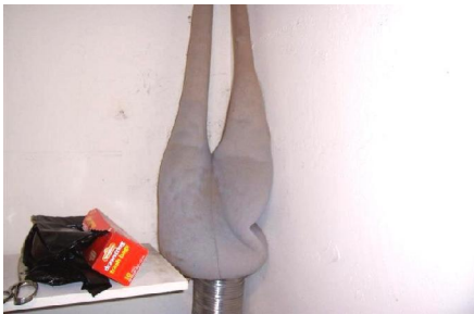
Figure 19. Non-standard dryer venting using a nylon stocking.
