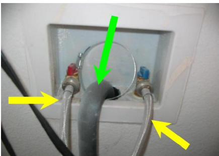
Figure 4. Metal braid water supply lines (yellow) and solid rubber drainage line (green) in use for the washer.
