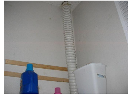
Figure 15. Long, vertical, corrugated plastic flue.
