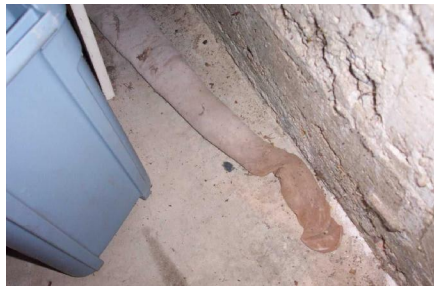
Figure 20. Non-standard dryer venting using a nylon stocking.
