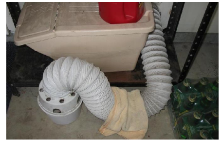
Figure 21. Non-standard dryer "wet vent."
