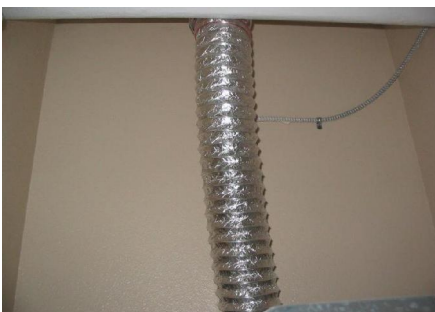
Figure 10. Corrugated metal foil dryer flue.
