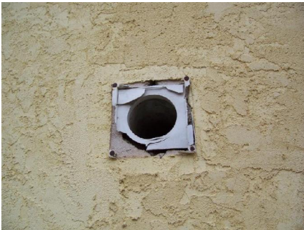
Figure 16. Missing dryer vent hood at exterior location.
