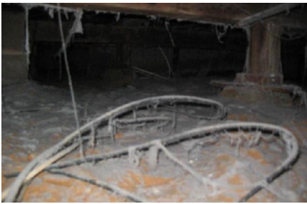
Figure 7. Accumulation of lint in the foundation crawl space.
