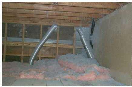
Figure 8. Accumulation of lint in the attic.
