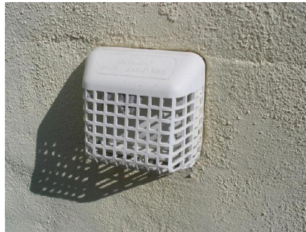
Figure 17. Protective device for the dryer vent hood.
