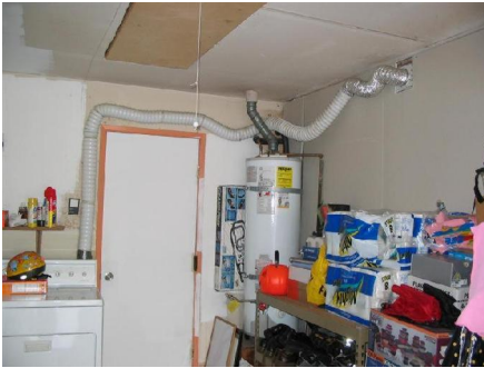
Figure 13. Excessively long combination corrugated plastic/metal dryer flue.
