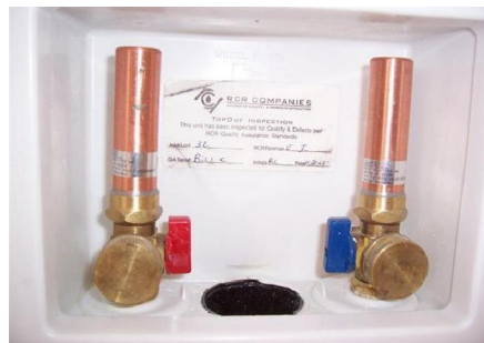
Figure 5. Water hammer arrestors installed at the laundry.
