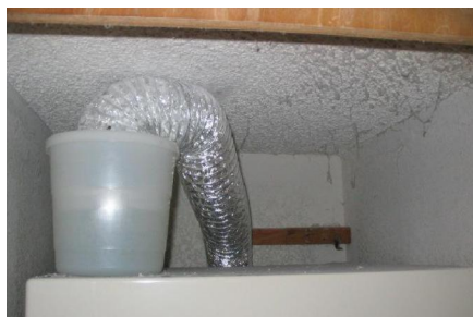
Figure 23 Non-standard dryer "wet vent."
