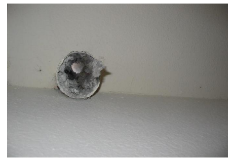
Figure 12. Clogged dryer flue.
