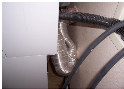
Figure 11. Corrugated metal foil dryer flue that has been crushed.
