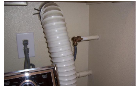
Figure 9. Corrugated plastic dryer flue.
