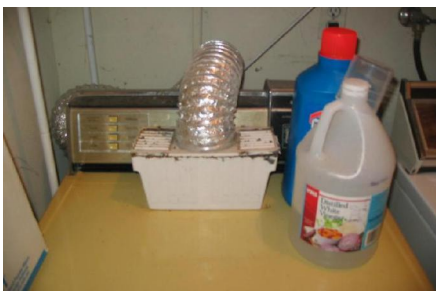
Figure 22 Non-standard dryer "wet vent."
