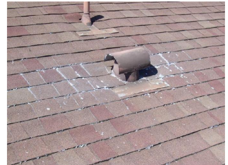
Figure 18. Lint accumulation on the roof.
