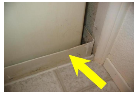
Figure 6. Drain pan under the washer.
