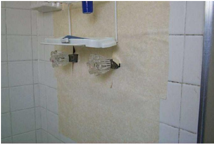
Figure 4. Improper tile and grouting repair.
