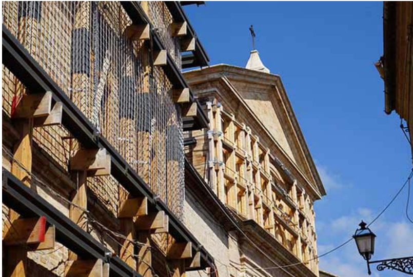
Figure 1. Reinforced buildings in Falerone after the earthquake, Váli, I., (2017)
