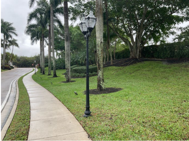
Light pole and fixtures
