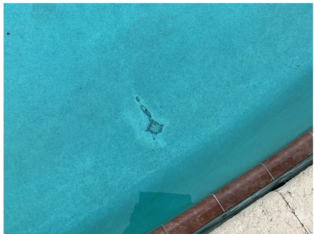
Plaster chips at pool
