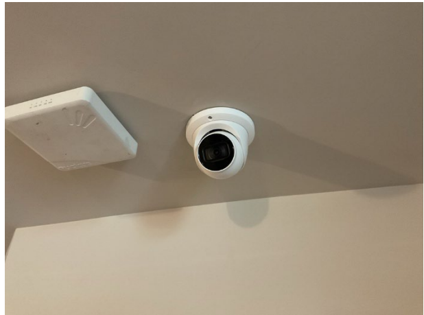
Security system camera
