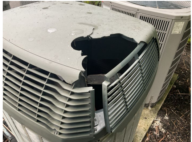
Damaged condensing unit
