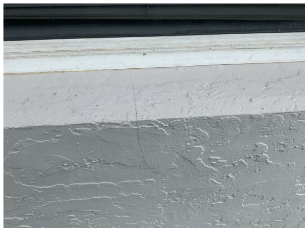
Stucco cracks at guardhouse
