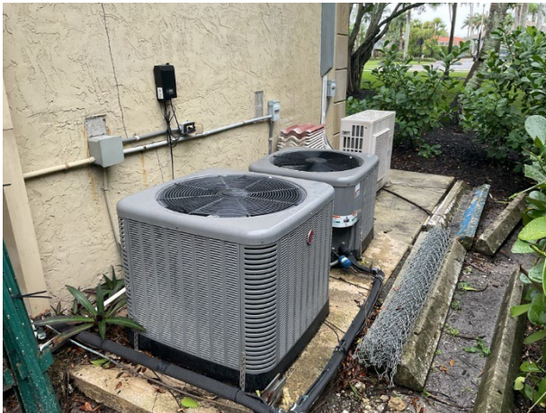
Split system condensing units
