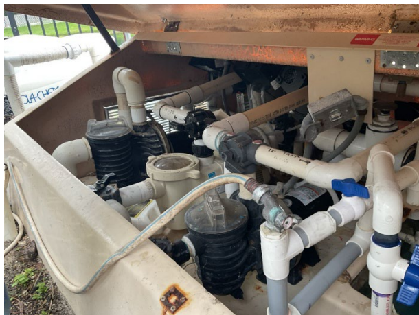
Pool pumps and filters
