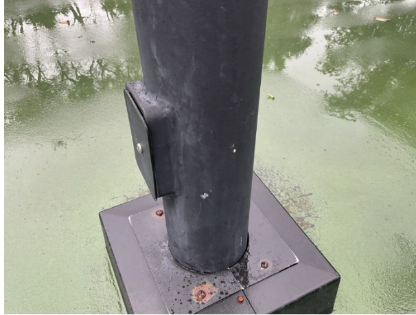
Pole finish deterioration
