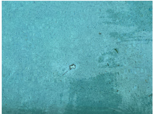
Plaster chips at pool
