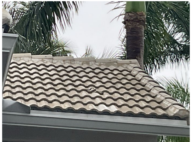
Damaged tiles at clubhouse
