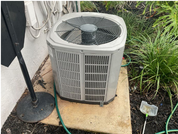
Split system condensing unit
