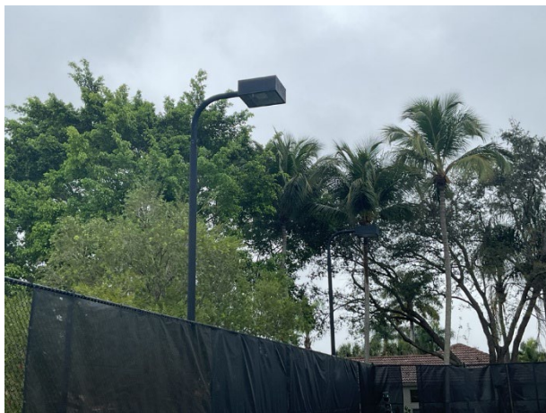
Light poles and fixtures
