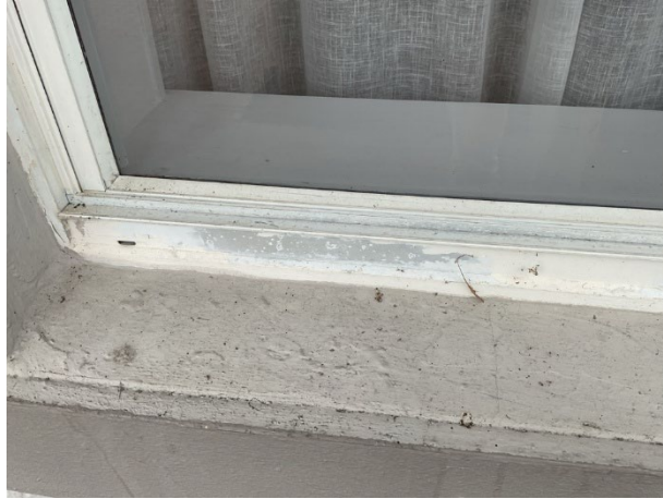
Frame finish deterioration
