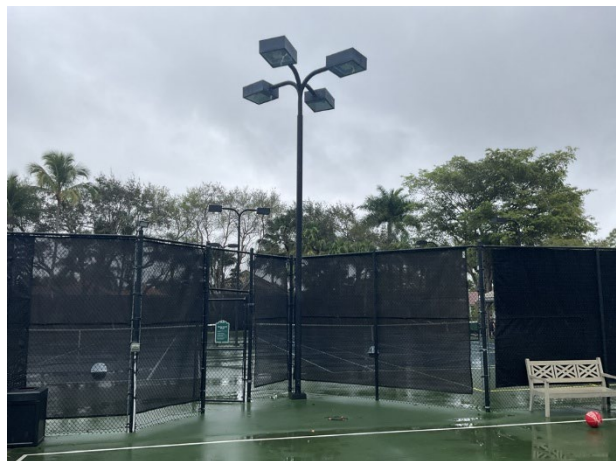
Light pole and fixtures
