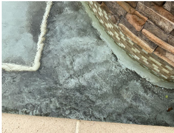
Plaster discoloration at fountain
