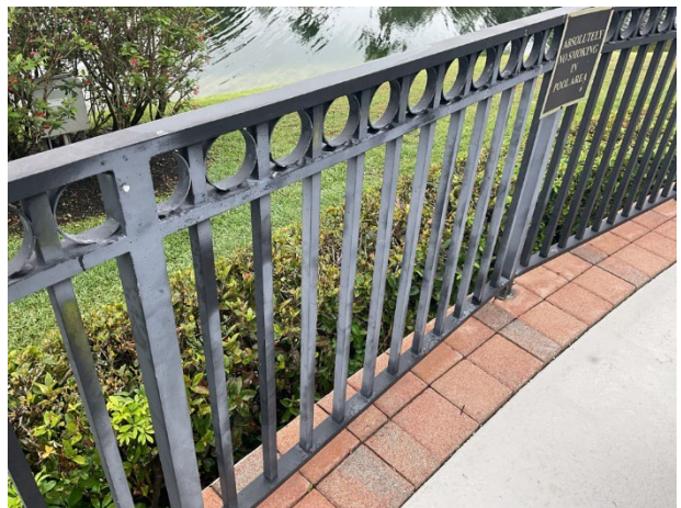
Fence finish deterioration
