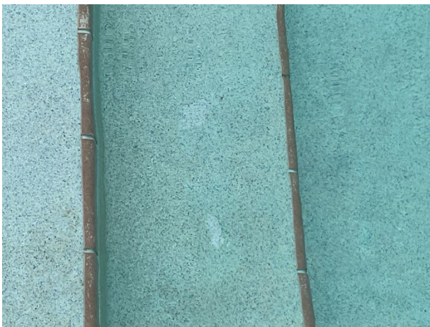
Plaster chips at pool
