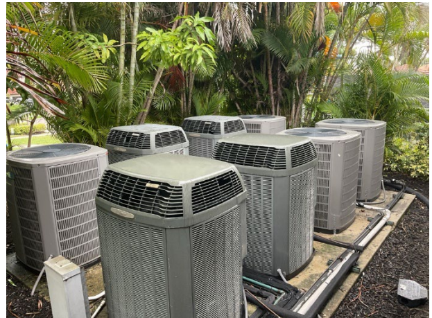
Split system condensing units
