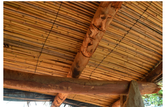
Reed is used as bottom layer in many roofs. Roof in Chome, Rumphu. © Jon Twingi.
