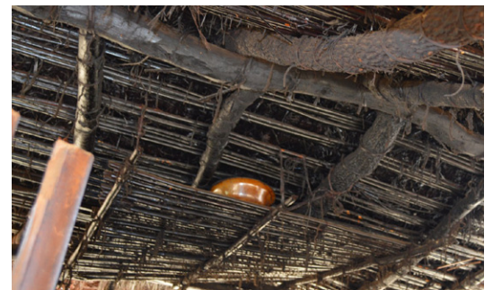
Raised platforms inside the houses are used to store food and seeds, preventing them to be damaged by floods. House in Chakhutupa, Chitipa. © Jon Twingi
