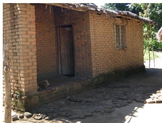
Raising dampness creates unhealthy living conditions inside the houses due to moisture. © Sonia Molina
