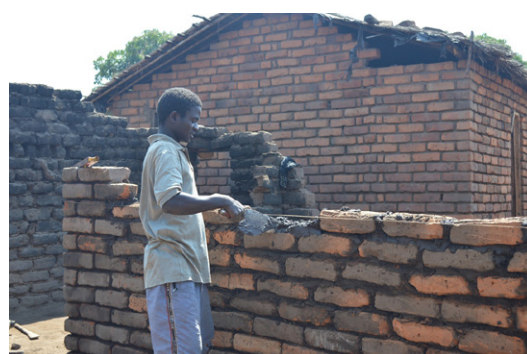
Burnt brick wall with cement mortar being built in Kambewa, Mulanje. © Jon Twingi.
