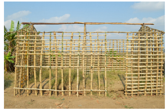
Light structures are good solutions in the event of an earthquake as even if they fall they are less likely to cause damages. Structure of a wattle and daub house in Mwaluwimba, Karonga. © Jon Twingi
