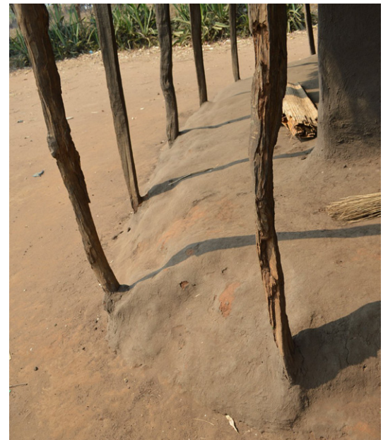
When wooden poles are in direct contact with the ground and are not regularly treated or replaced, they are vulnerable to rising damp and decomposition. Veranda in Lifidzi, Salima. © Jon Twingi
