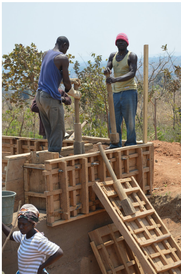
In some areas, there is a need to help one another build their home. Construction of a rammed earth house in Nisanje, Lilongwe. © Jon Twingi
