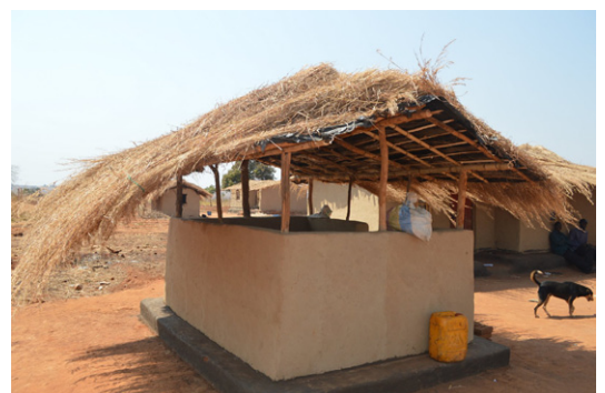
Kitchen with the upper parts of the walls open for improved ventilation. Nkhombe, Kasungu. © Jon Twingi
