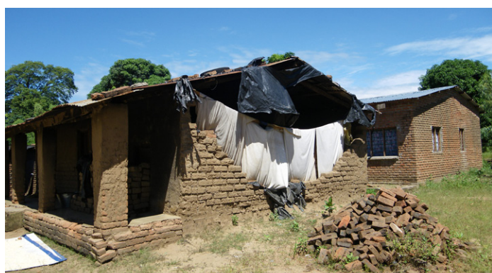
Unsupported masonry gables tend to fail in the out-of-plane direction in the event of an earthquake. This house's gable fell after the Karonga earthquake in 2009. © Sonia Molina
