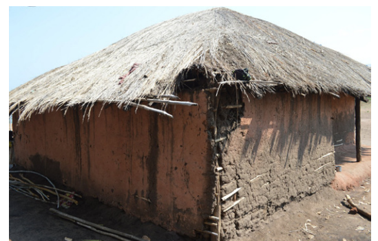
Maintenance of roofs is crucial to block water from penetrating the walls and to make them stay stable. House in Mwamwiyo, Karonga. © Jon Twingi
