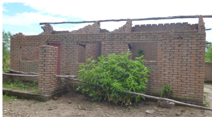
CGI sheets roofs can easily be blown off at high speeds in the event of strong winds creating an important risk. When the roof of the veranda is not separate from the roof of the main structure, the uplift of the entire roof can more easily happen. House in Karonga. © Sonia Molina
