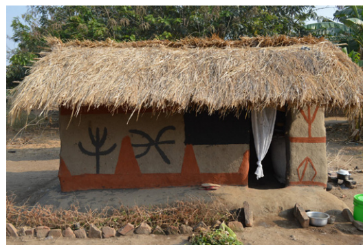
Flexible structures like wattle and daub ones better accept the deformations resulting from ground movements. Also, limited dimensions of constructions help avoid important crackings. Wattle and daub house in Malengamzona, Karonga. © Jon Twingi
