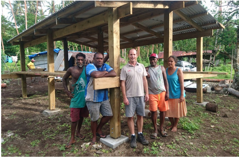
Fig. 8: A house structure was provided in the government shelter project in Maewo, which the beneficiary was expected to complete (source: Daily Post, 2019).
