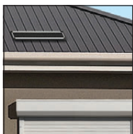
Roof Mounted Unit
