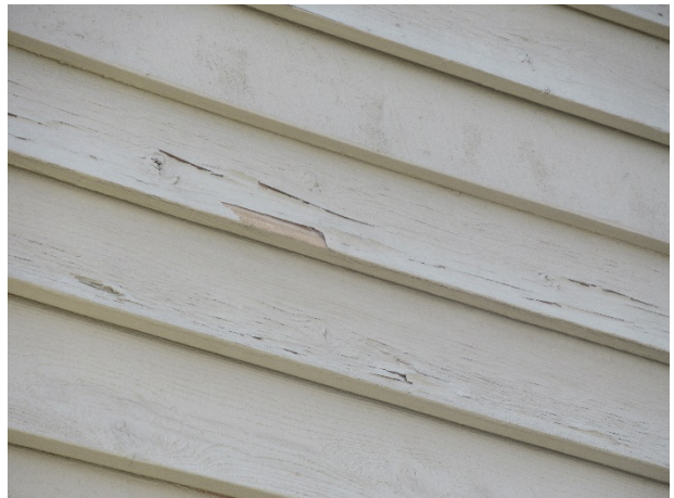
Paint finish deterioration (27W202 shown)
