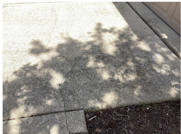
Driveway cracks (0N671 shown)
