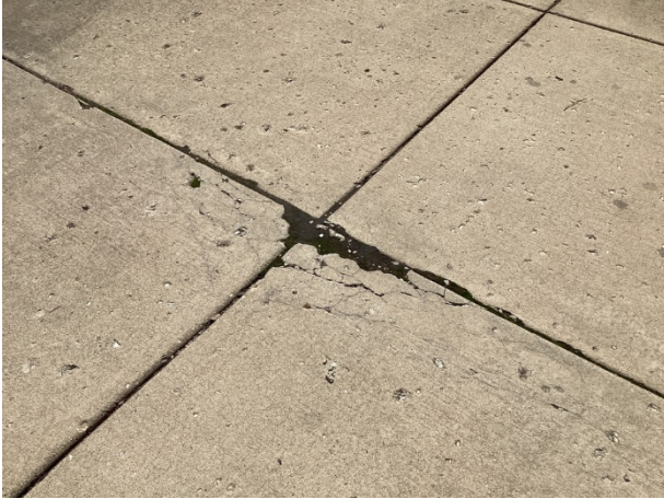
Driveway cracks (0N674 shown)
