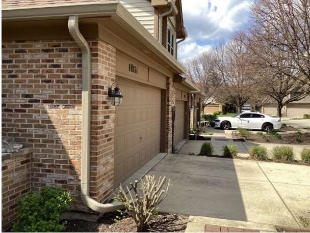
Exterior light fixture
