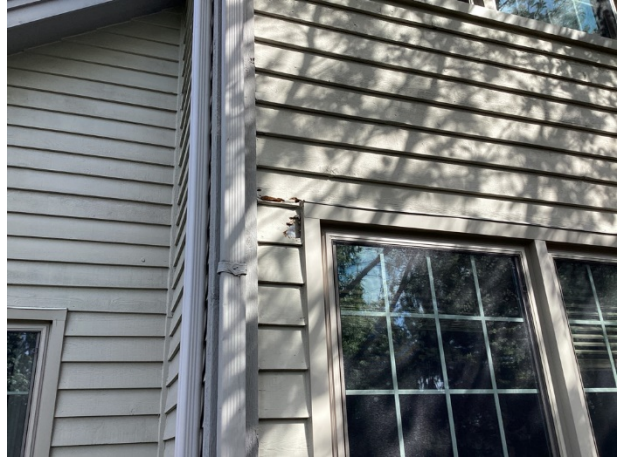
Siding damage (0N684 shown)
