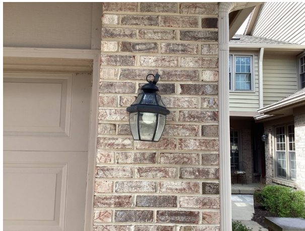
Fixture damage (27W234 shown)
