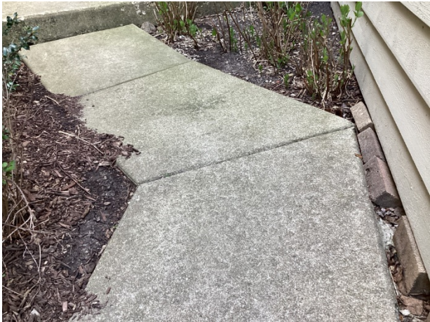
Sidewalk settlement (0N675 shown)
