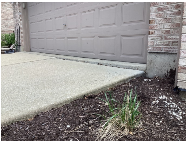
Driveway settlement (0N679 shown)
