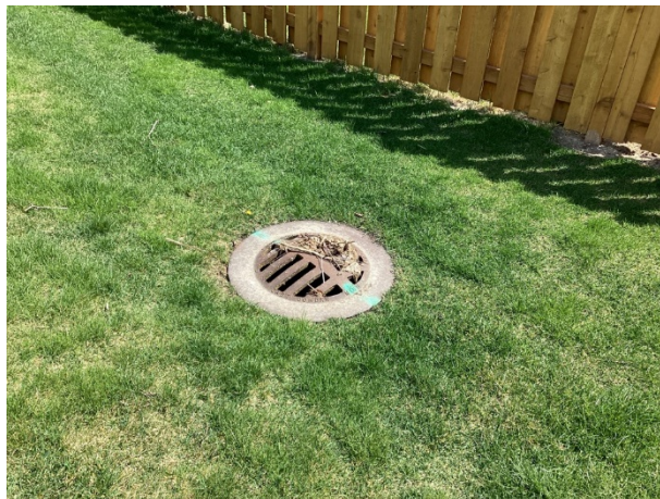
Debris accumulation at catch basin
