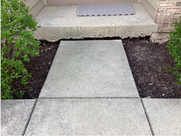
Sidewalk settlement and stoop undermining
