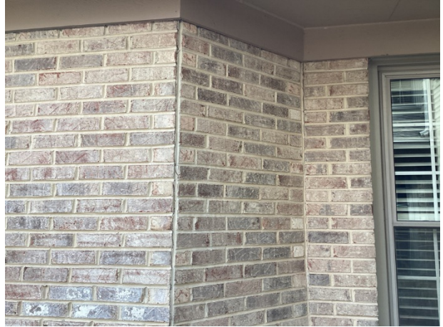
Mortar cracks (27W234 shown)
