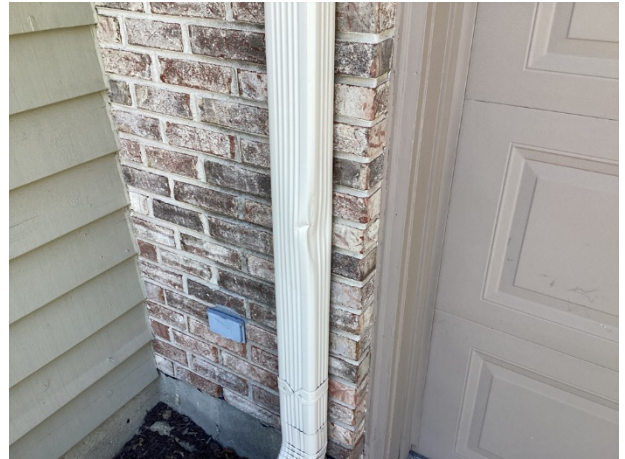
Downspout damage (27W224 shown)
