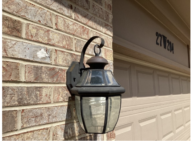
Fixture finish deterioration
