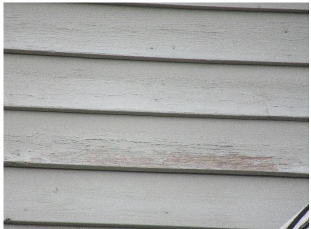
Paint finish deterioration
