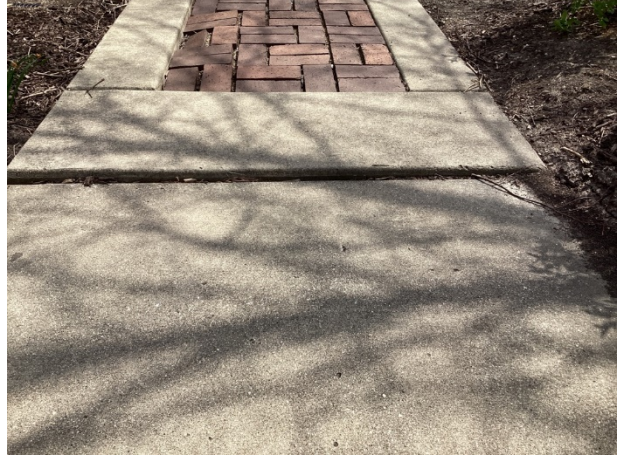
Sidewalk trip hazard (0N677 shown)
