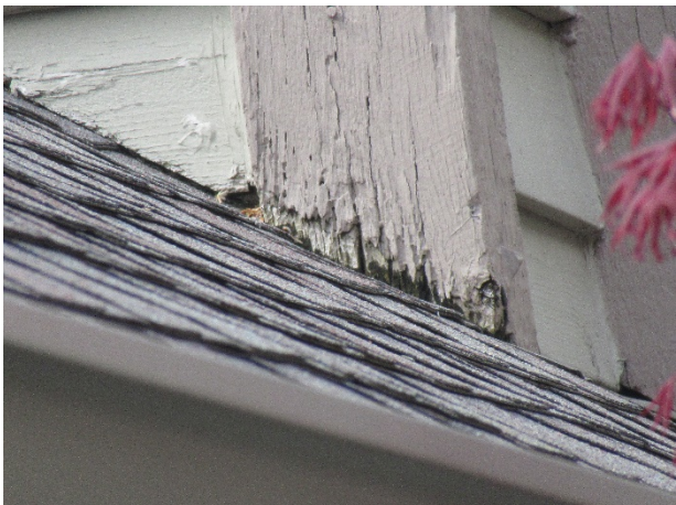
Siding in contact with roof (27W202 shown)
