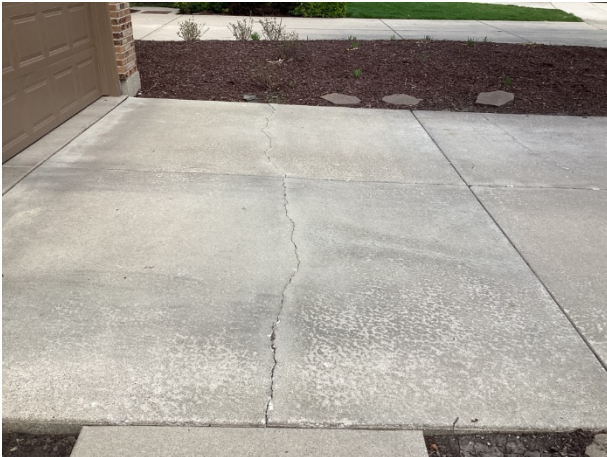
Driveway cracks (27W216 shown)
