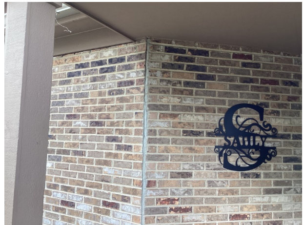
Mortar crack (27W212 shown)
