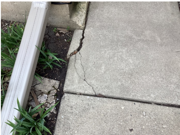
Sidewalk cracks (0N674 shown)
