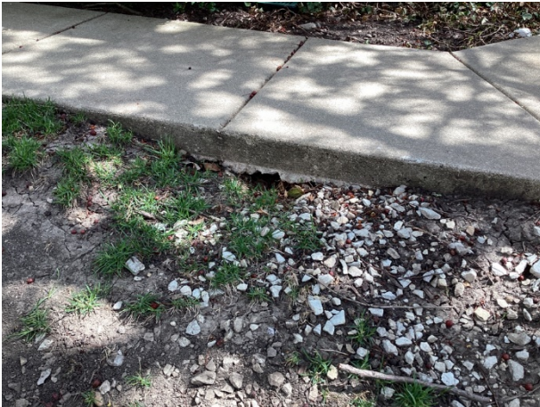
Soil undermining at sidewalk (0N667 shown)
