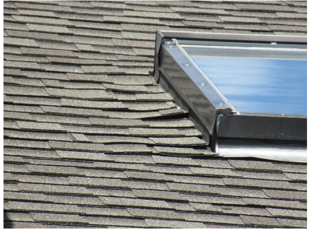
Shingle lift at skylight (27W204 shown)
