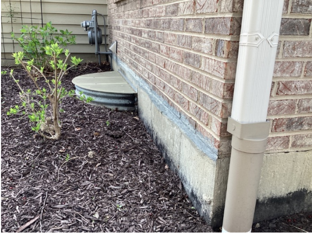
Improper masonry patch (27W224 shown)
