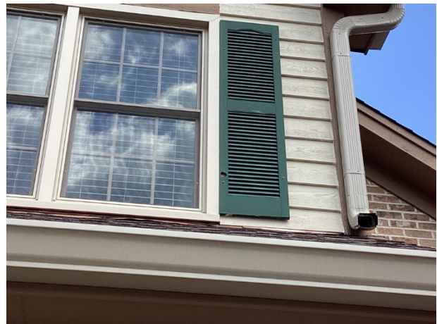
Shutter damage (0N673 shown)
