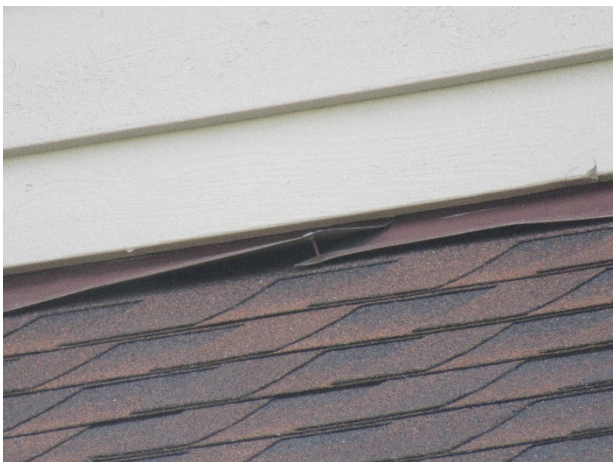
Nail pop at flashing (0N698 shown)
