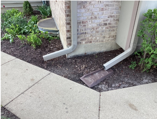
Improper downspout runoff
