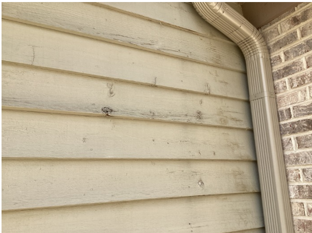
Siding deterioration (27W202 shown)
