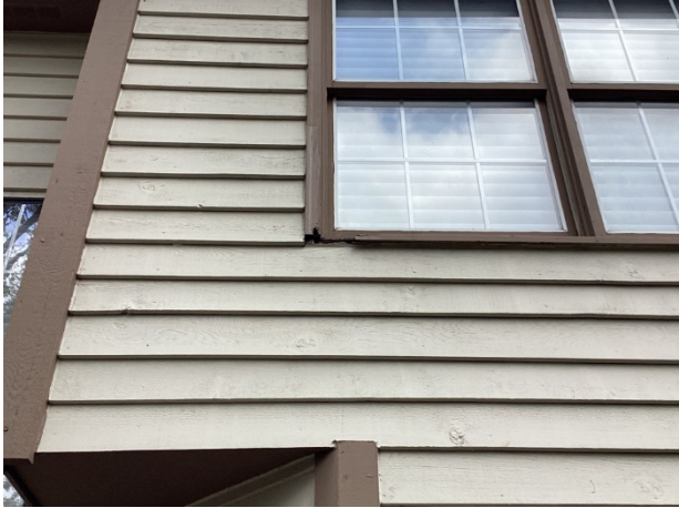
Window trim damage (0N685 shown)
