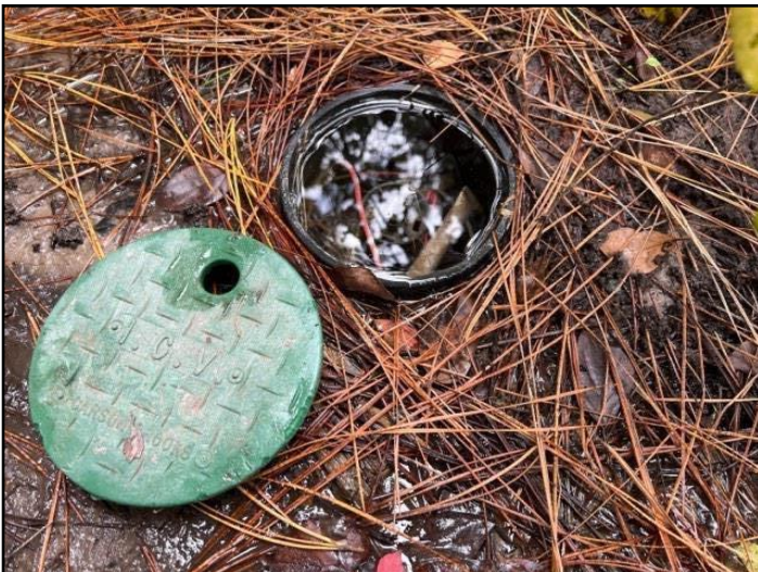
50. Water inside ICV for sprinkler
