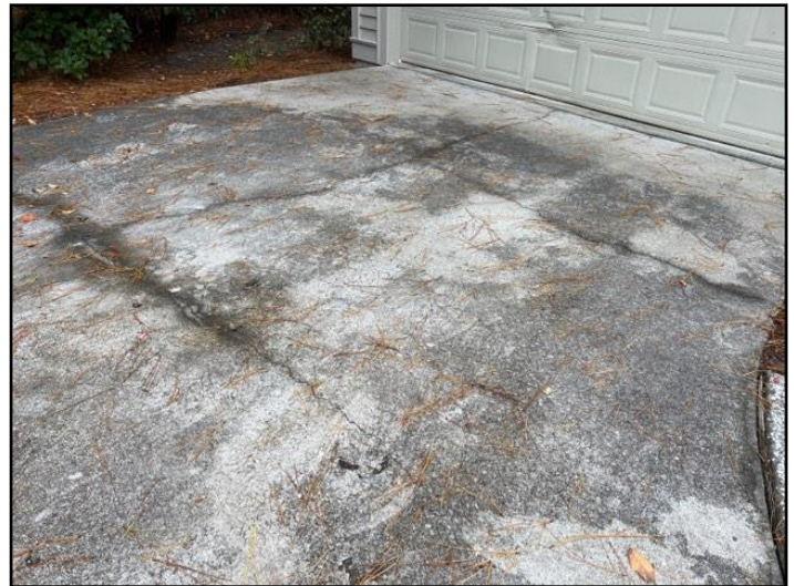
43. Minor cracking on driveway
