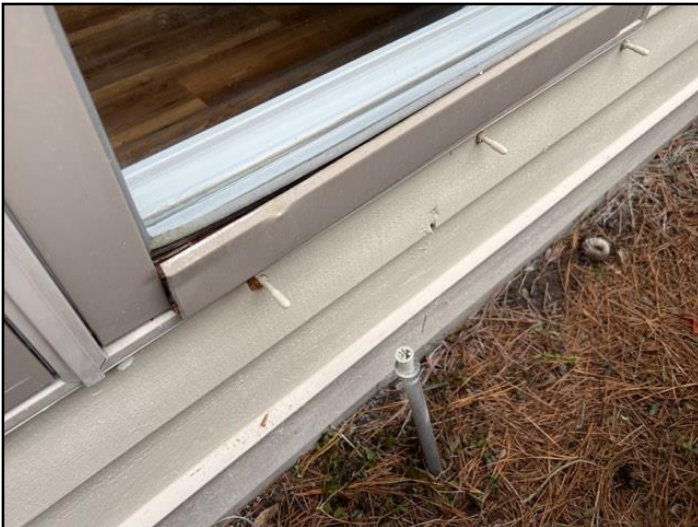
1. Loose metal trim at window
