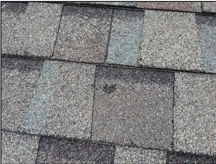
14. Minor impact damage
