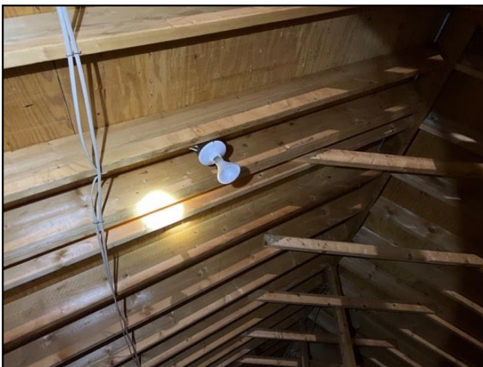
90. Inoperative lights in attic
