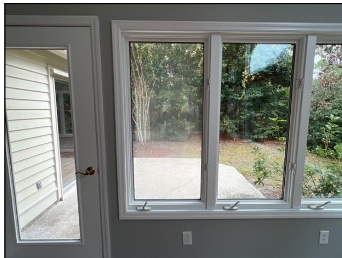
171. Fogged Glass on window in sunroom
