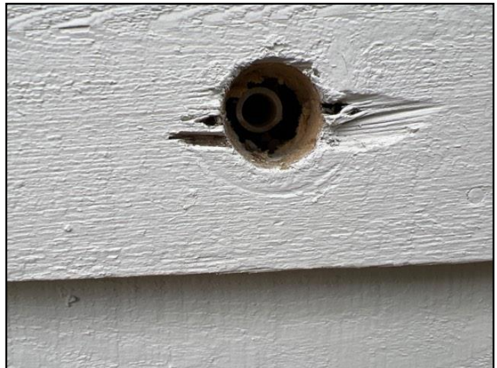
30. Open gap w/ old piping
