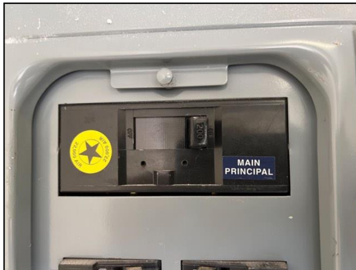
71. 200 Amps Main disconnect
