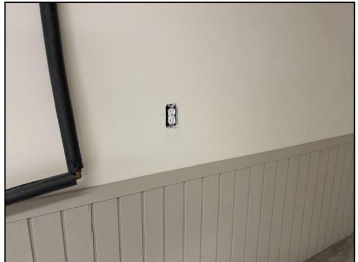
84. Missing cover plate at receptacle
