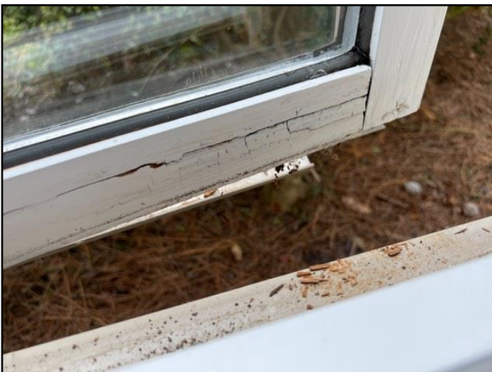
3. Interior lower rail damaged
