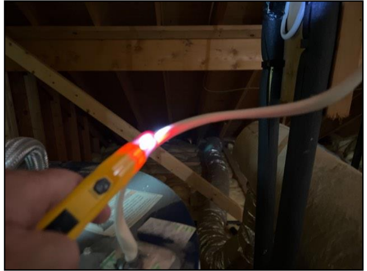
133. Live wire to water heater.
