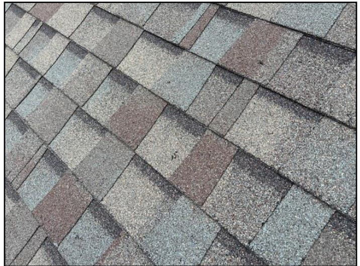
15. Minor impact damage
