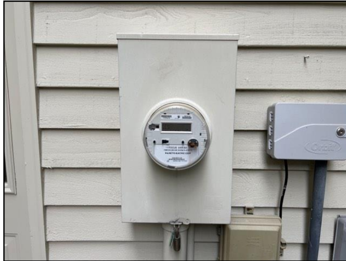
70. Underground aluminum at meter
