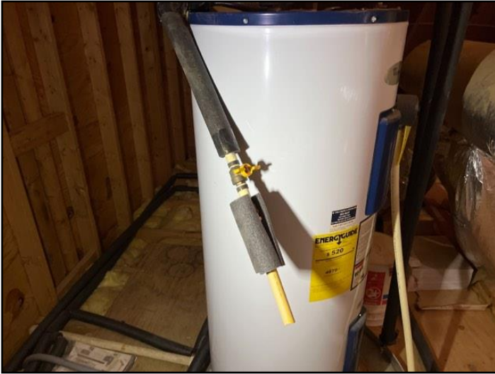
132. No water supply attached
