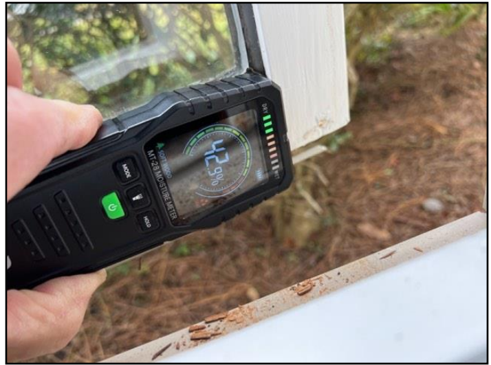
36. Moisture present at window
