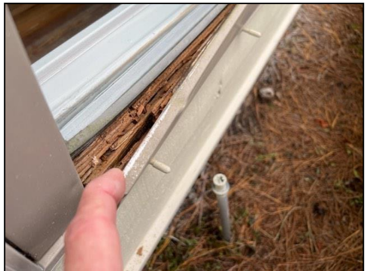
34. Wood deteriorated behind metal trim
