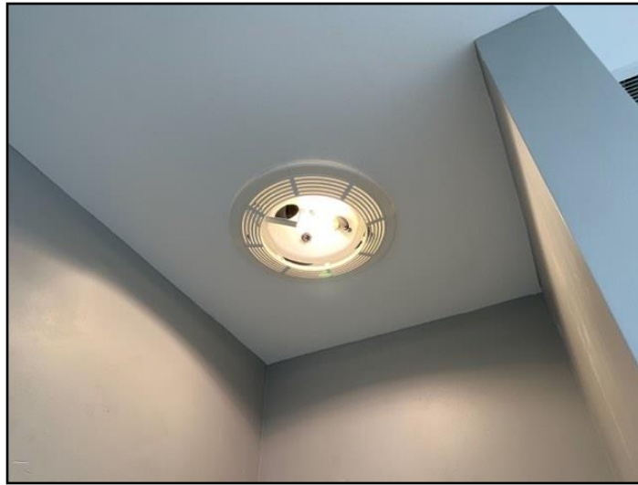
92. Missing lens cover at light/vent fan
