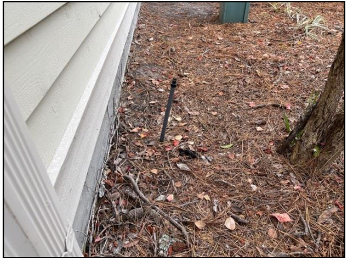
55. Tilted sprinkler heads
