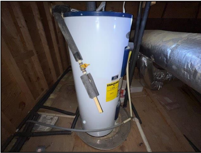
143. Inoperative water heater
