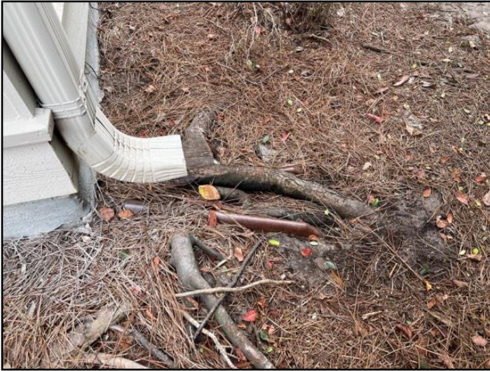
27. Minor soil eroding below gutter discharge
