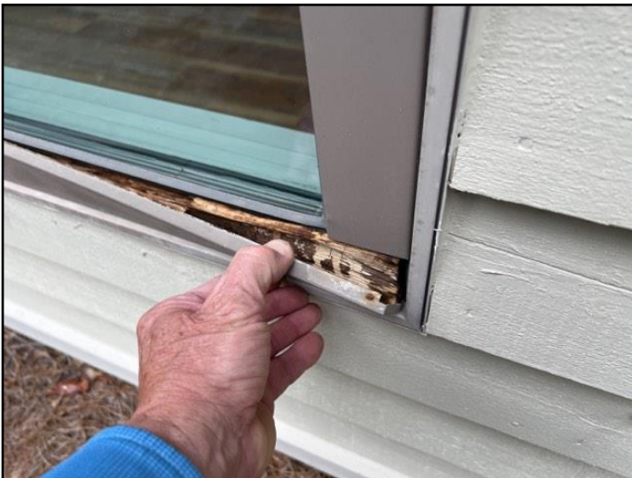
37. Wood deteriorated behind metal frame
