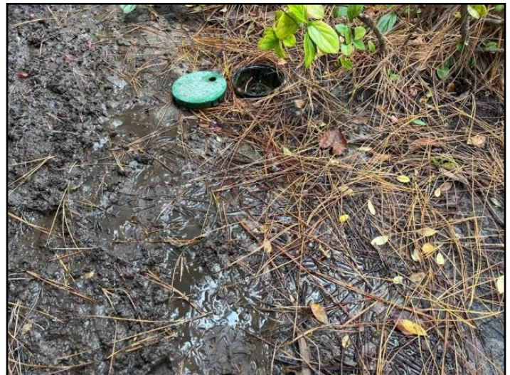
51. Ponding of water along garage wall
