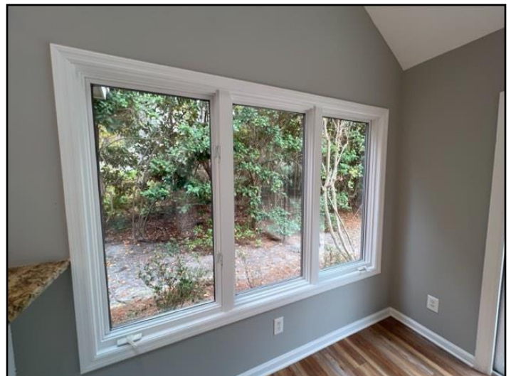
174. Missing screens an windows
