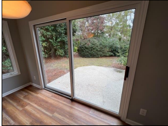
175. Glass slider difficult to open
