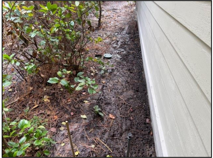
53. Ponding of water along garage wall
