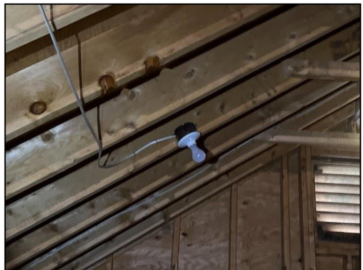
91. Inoperative lights in attic
