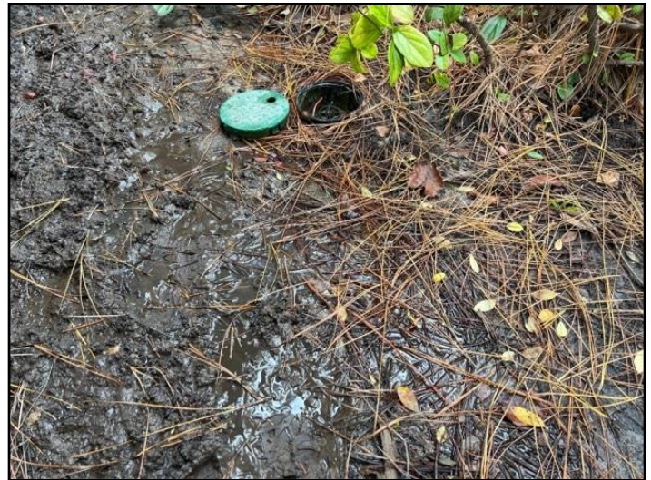
9. Ponding of water along garage wall
