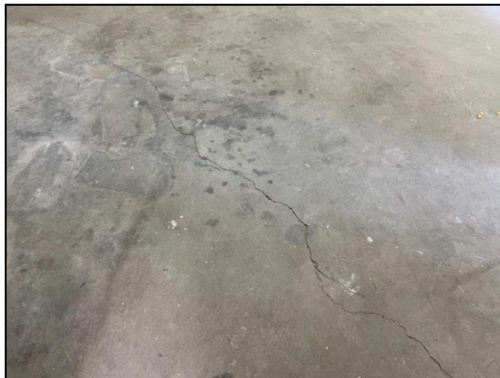
176. Minor crack on garage floor
