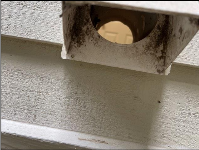
31. Dryer vent missing flapper
