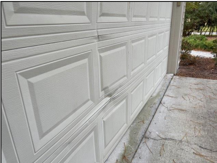
46. Dented garage door
