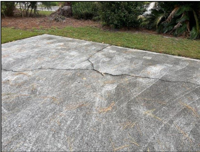
42. Minor cracking on driveway
