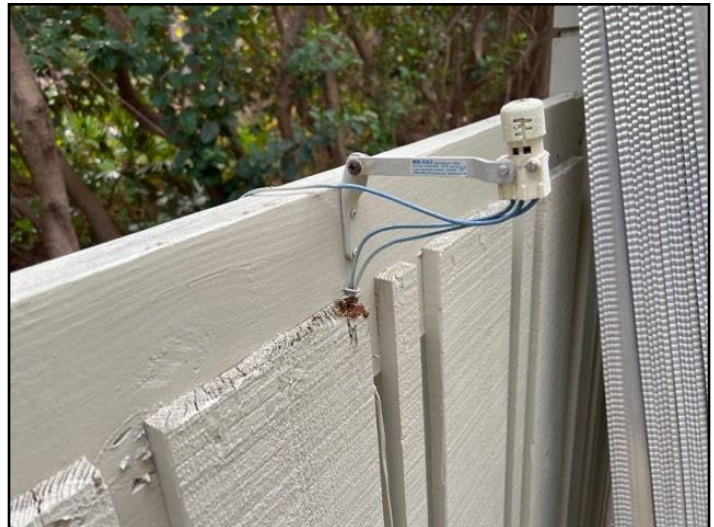
45. Minor deterioration to fence boards
