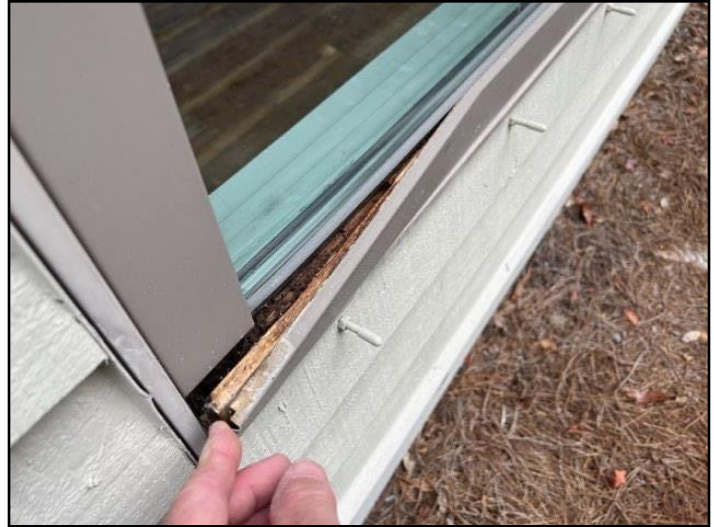
6. Wood deteriorated behind metal frame
