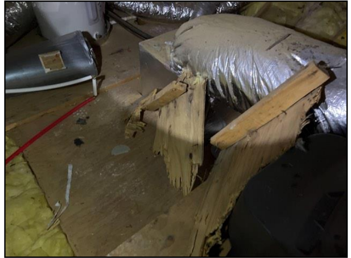
122. Debris in attic
