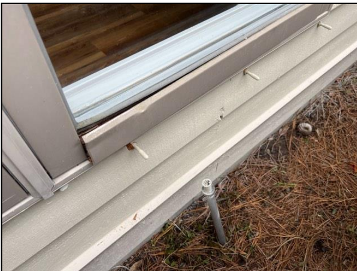
33. Loose metal trim at window
