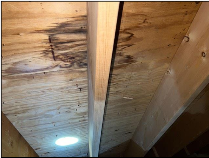
68. Water stains on rear sheathing
