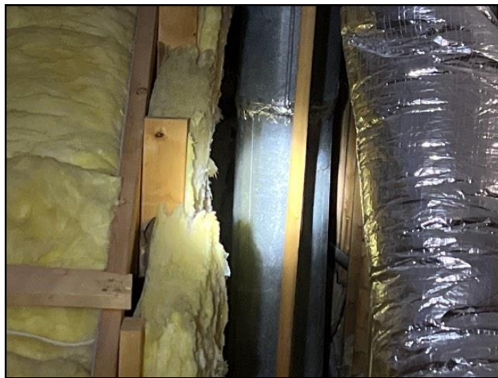
99. Metal vent piping in attic
