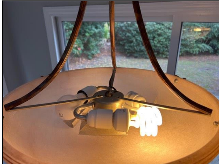
87. Bulbs out at light in kitchen
