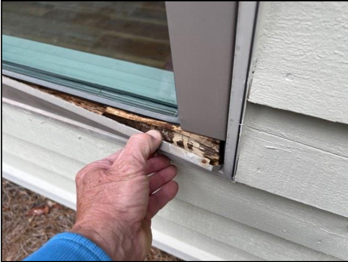
5. Wood deteriorated behind metal frame
