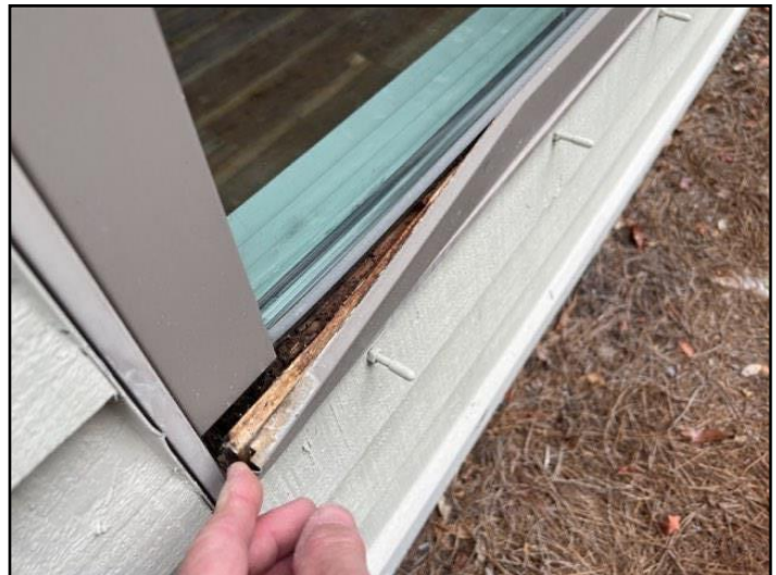
38. Wood deteriorated behind metal frame
