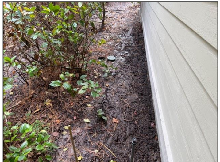
11. Ponding of water along garage wall
