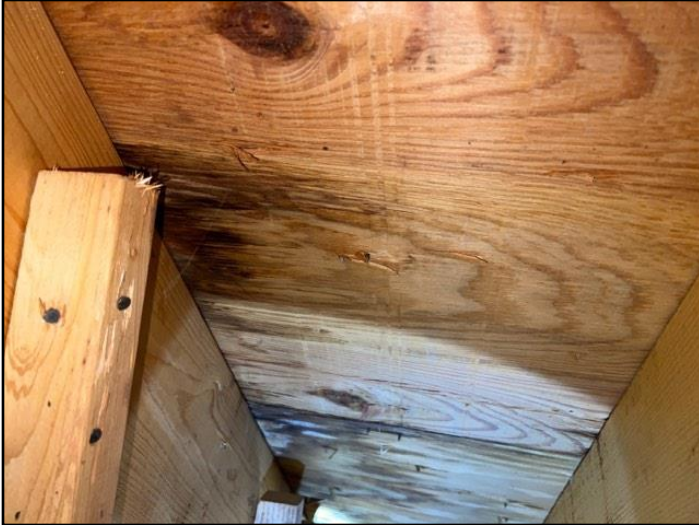
64. Water stains on door sheathing, garage
