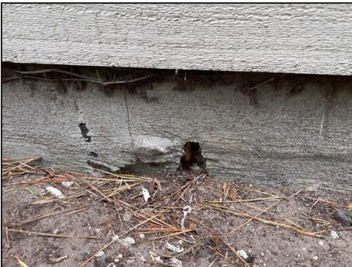
62. Typical minor cracks at slab
