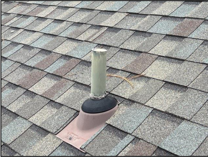
136. Plastic on roof
