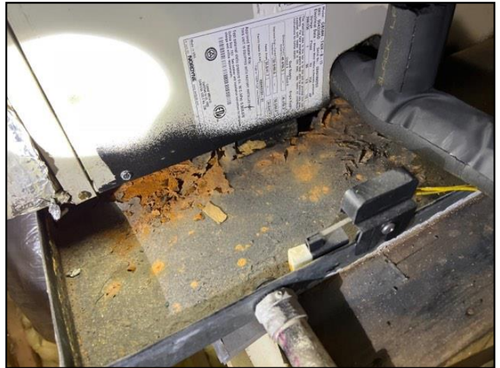
115. Rust in pan
