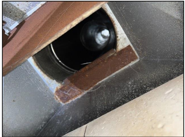
94. Metal flue operational
