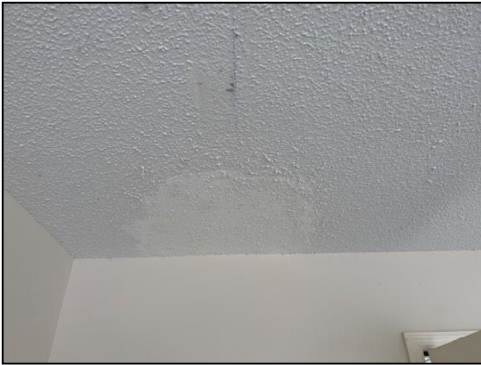
167. Patched ceiling in garage
