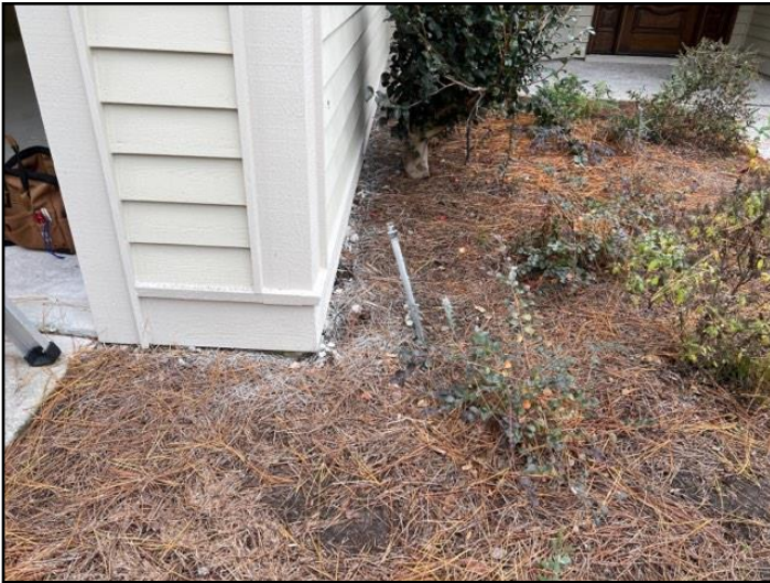
54. Tilted sprinkler heads
