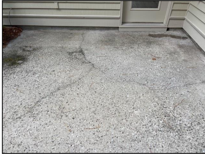
41. Minor Cracking on rear patio
