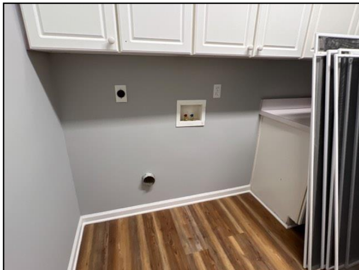
161. No washer or dryer in laundry room.
