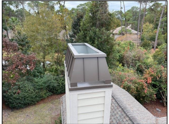
98. Metal chimney shroud
