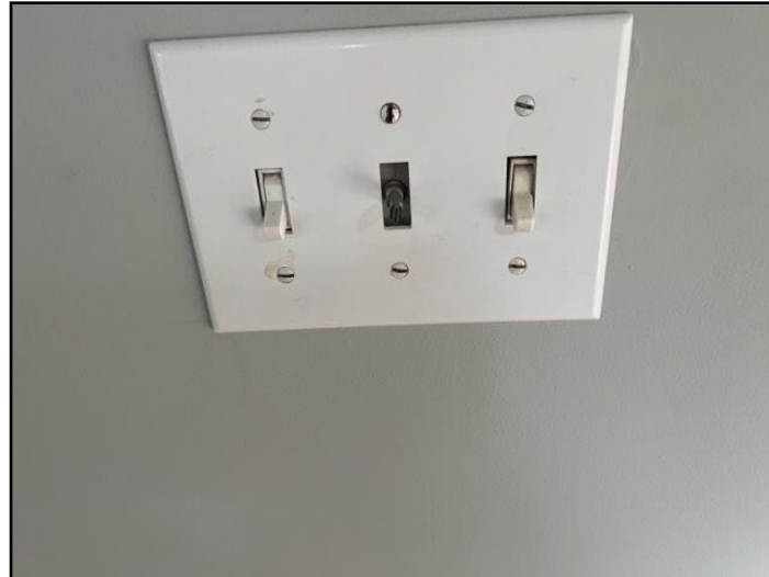
82. Rotary knob missing at light switch
