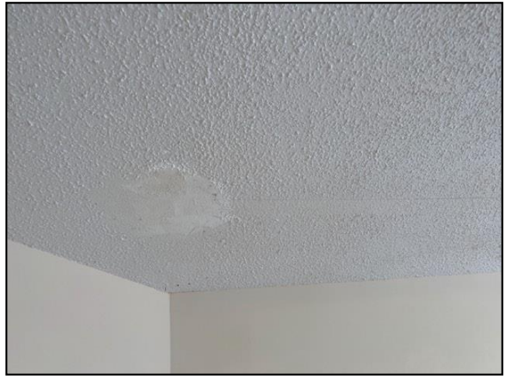
168. Patched garage ceiling
