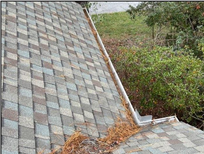
25. Clogged gutters, front
