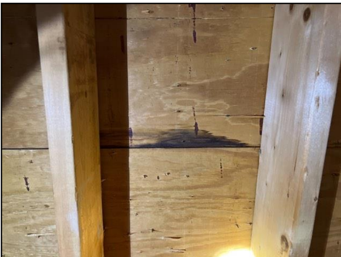
66. Water stains on roof sheathing
