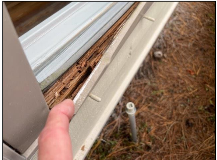
2. Wood deteriorated behind metal trim
