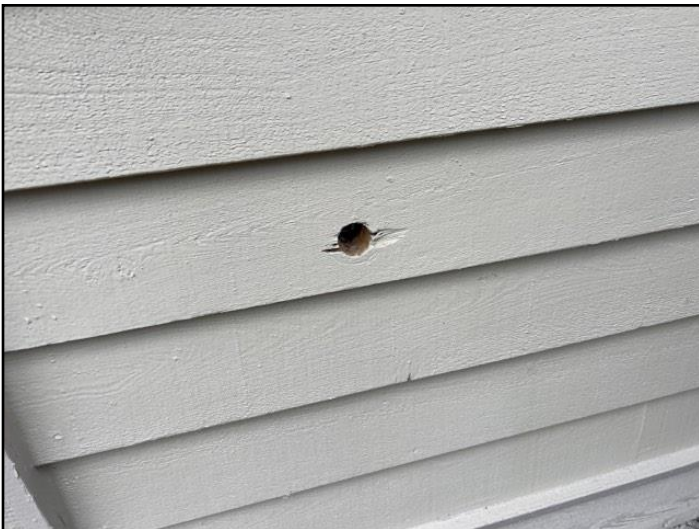
29. Open gap in siding
