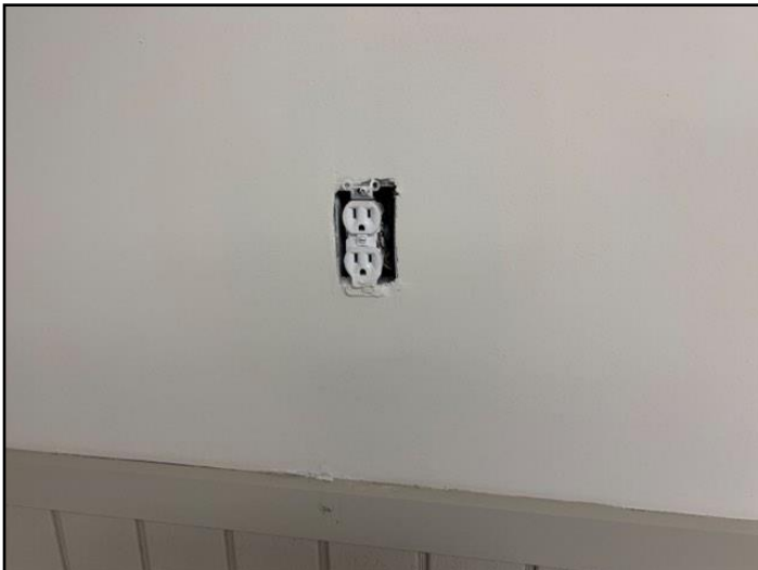
83. Missing cover plate on outlets in garage
