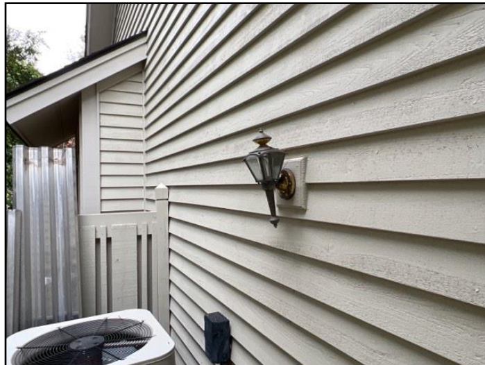
86. Inoperative light at service area.
