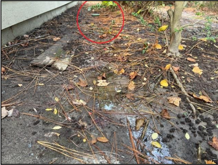
52. Ponding of water near ICV
