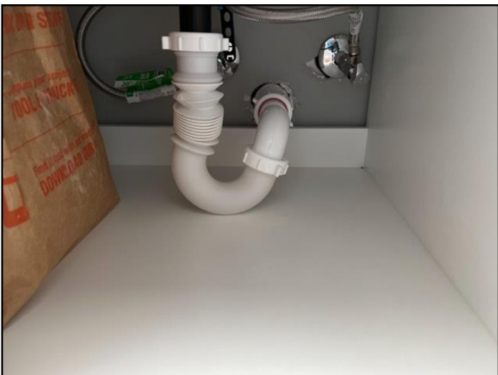
148. Flexible accordion waste piping
