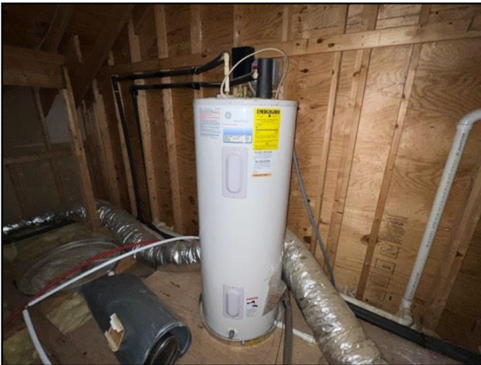
126. General Electric water heater
