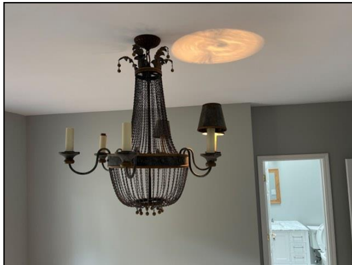
88. Bulbs missing at light fixture
