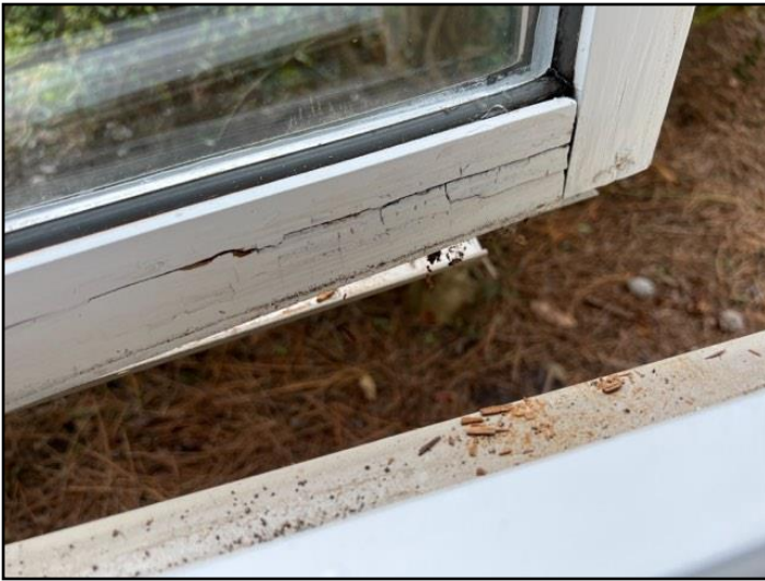
35. Interior lower rail damaged
