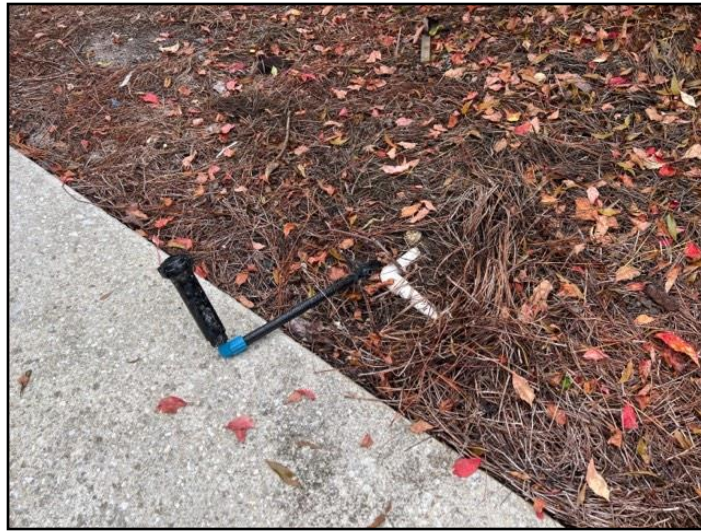
56. Exposed piping and loose sprinkler head
