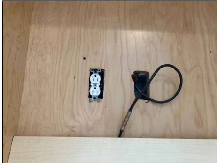
85. Missing cover plates
