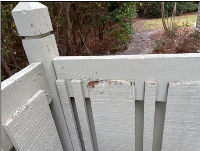
44. Minor deterioration to fence boards
