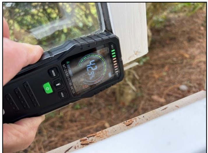
4. Moisture present at window
