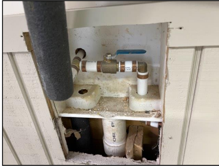
125. Main water shut off Garage.
