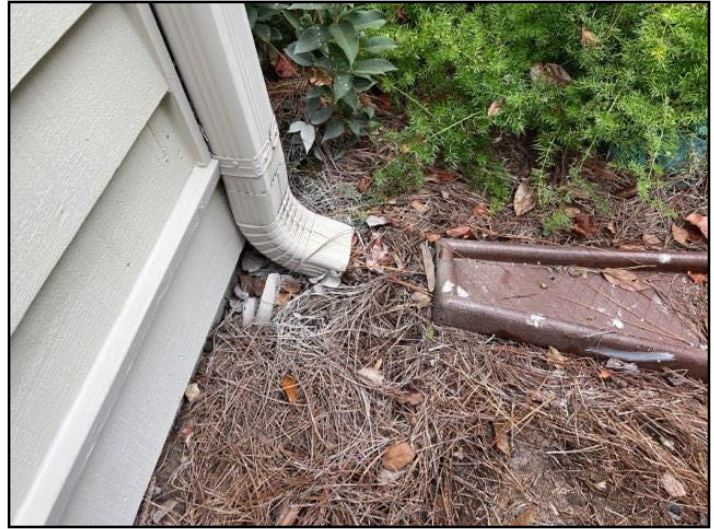
28. Discharge covers with debris
