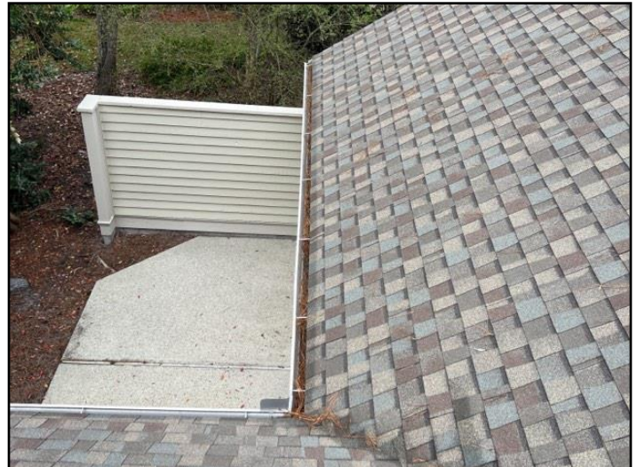
26. Clogged gutters, rear
