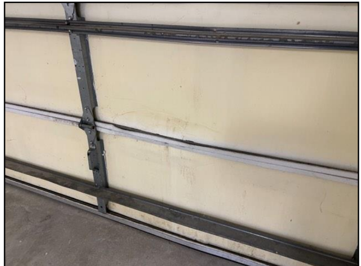
47. Dent viewed from inside garage
