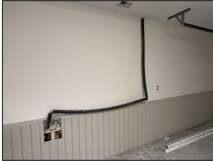
140. Supply piping loose in garage
