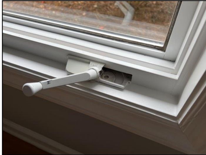
172. Broken cover at hand crank mechanism
