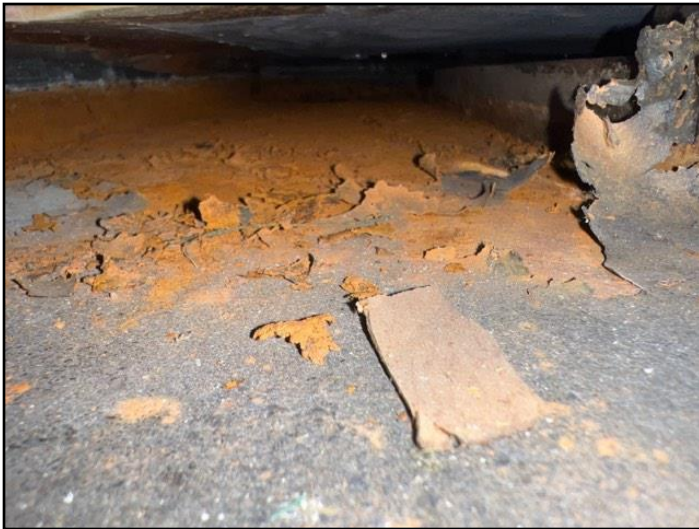
114. Rust in condensate pan
