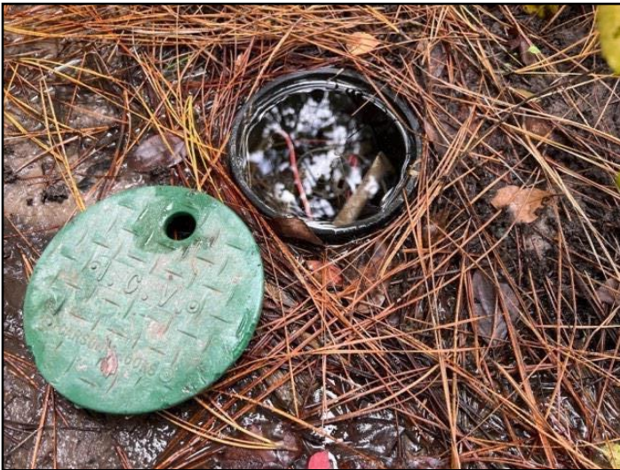
8. Water inside ICV for sprinkler
