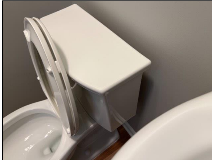
151. Loose tank on top of toilet base
