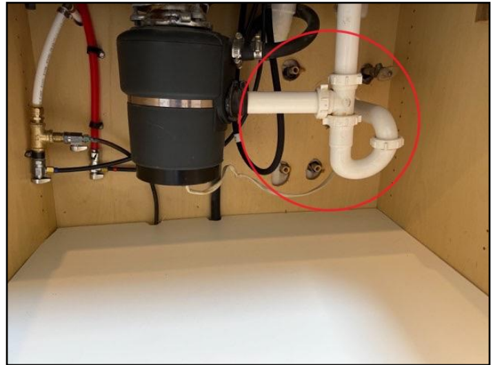
142. Older abandoned supply lines
