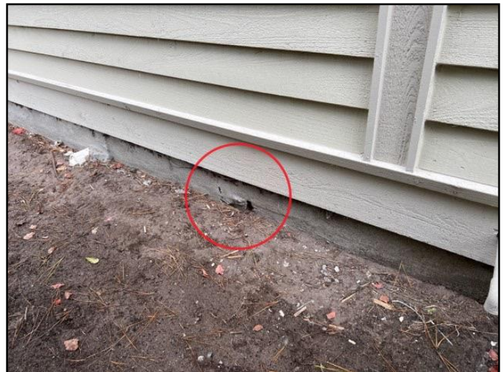
63. Typical minor cracks
