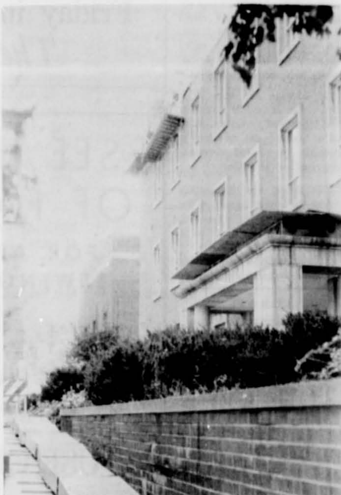
An error in roof design is responsible for the repair work presently being performed on the Roy O. West Library. Pressure caused by too few expansion joints is causing the top stone work to crack.
