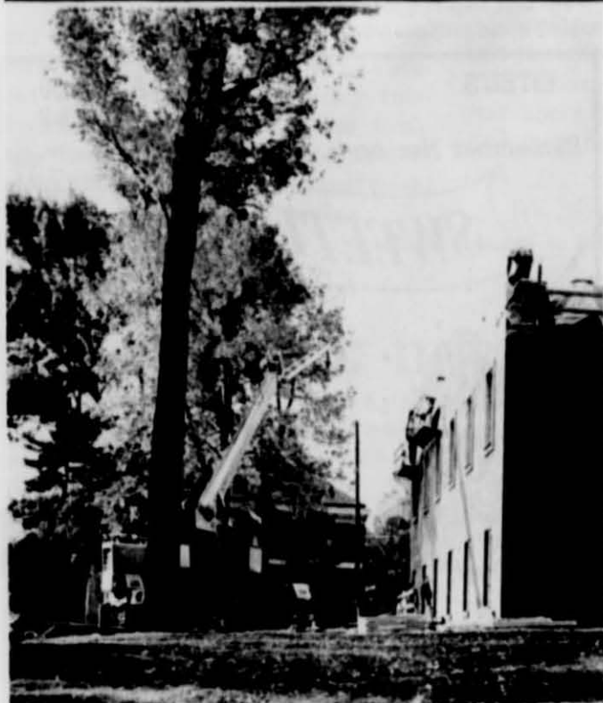
Repair work on the Roy O. West Library roof should be completed within two weeks, according to Bruce Collins of DePauw's maintenance department. The rear lower section of the roof is still being worked on.
