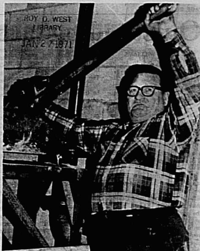
Bill Mellow, an Indianapolis plumber, works on the $4.5 million science center. Additional photos, page 6.
