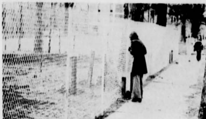
A fence was put up Wednesday between the Performing Arts Center construction site and the Locust Street sidewalk, causing conversational difficulties for Sally Herr and a near-invisible listener on the other side.
