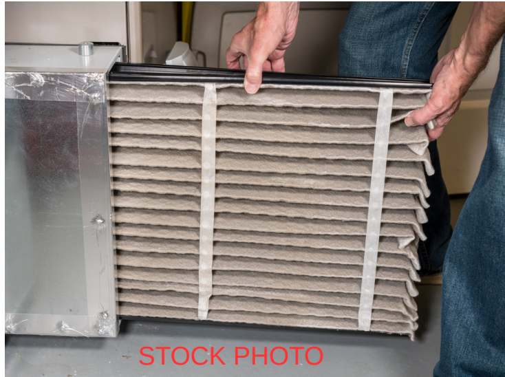
Observed dirty HVAC filter. Recommend replacement. Filter Size: 16x25x1
