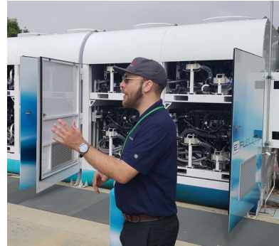
Perzynski reviews the capabilities of the stationary fuel cell power station
