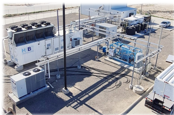
Aerial View of SoHyCal Hydrogen Production Facility
