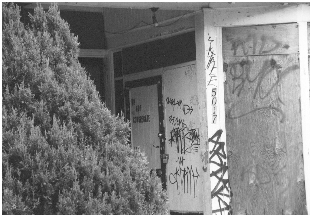
Photo 5: A vacant house on an otherwise occupied residential block in Frankford. It appears well sealed but the warning “Do don’t congregate” and the graffiti are visual evidence of the impact a single vacant house can have on a block. This house is less than one block from Frankford Hospital. Photo taken September 2001.
