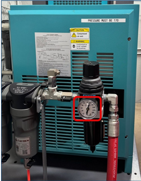
Figure 31. The compressor regulator gauge (boxed), on the side of the dryer behind the cutter. The white arrow sticker on the dial marks the target; 160 to 180 PSI is the range.
