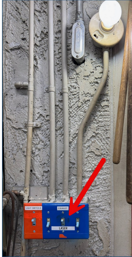
Figure 8. The roof exhaust fan switch is the middle toggle labeled LASER (arrow), by the doorway. The bulb above it lights when the fan is on.
