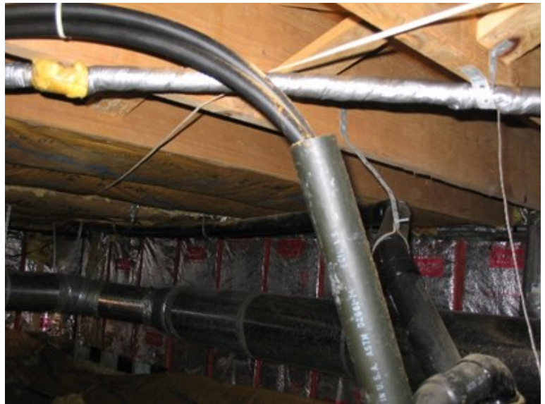
Direct connections between water filtration systems and sewers are not uncommon and pose a cross-contamination hazard.
