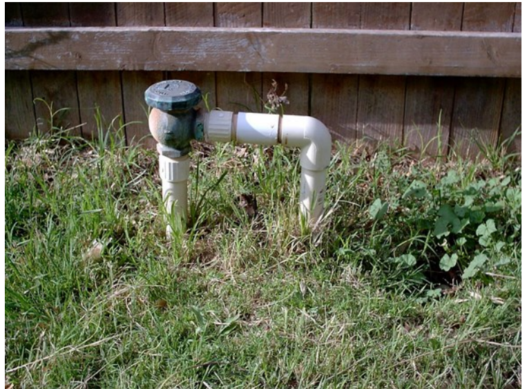
Atmospheric vacuum breakers are commonly used for sprinkler systems.
