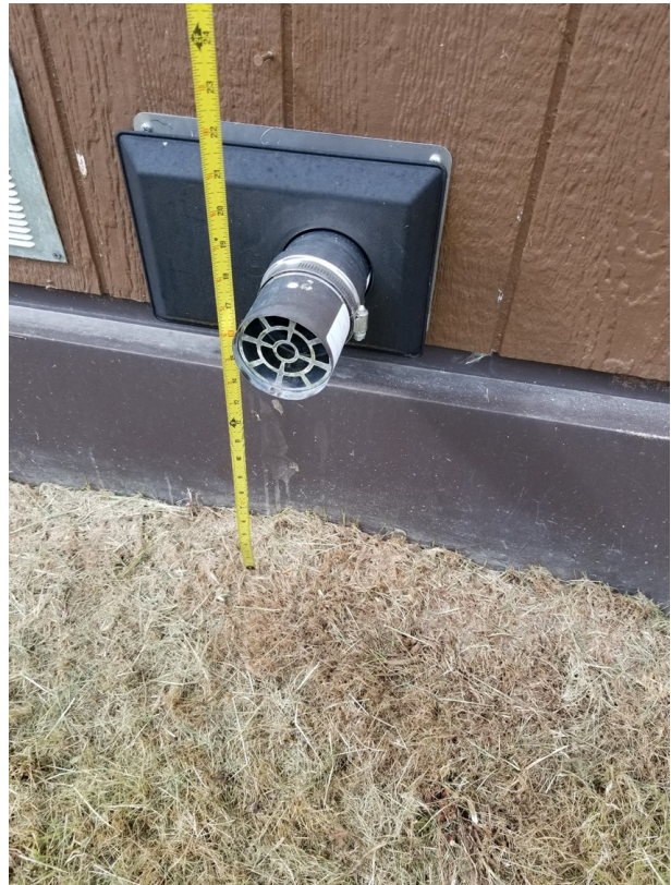
Exhaust too close to grade, subject to snow closure.
