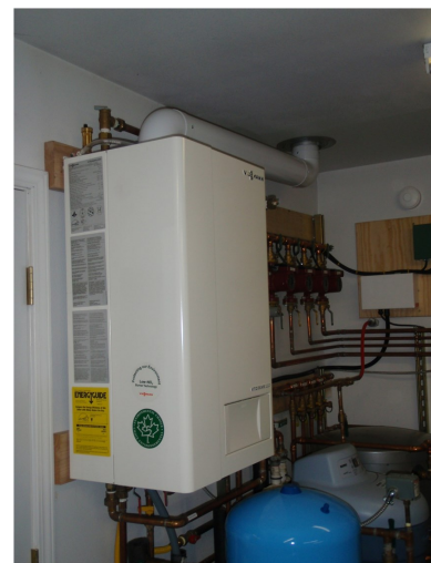
Sealed Combustion Appliance
