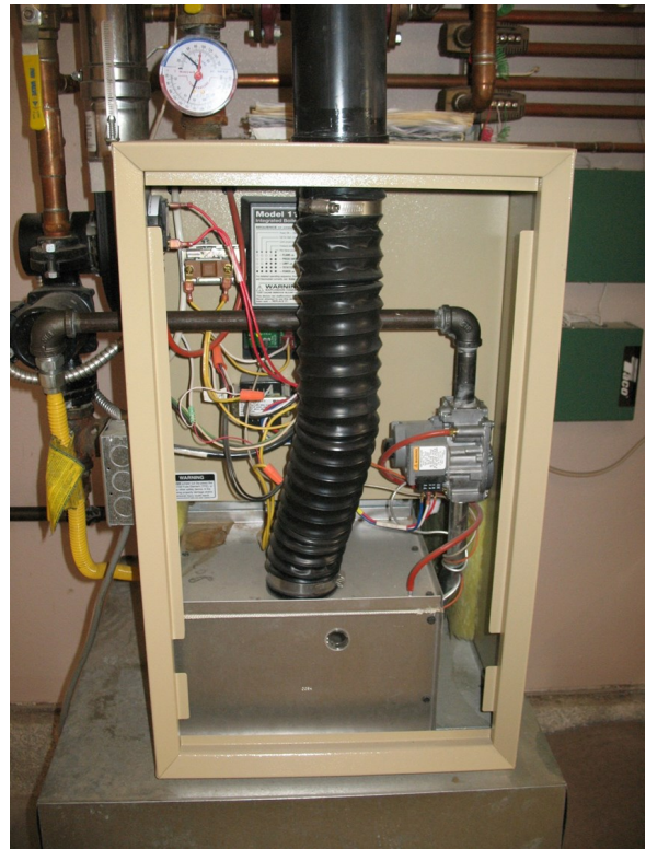
A Category 3, sealed combustion, non-condensing boiler.
