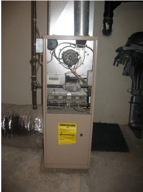
A Category 1, fan assisted draft, open combustion forced air furnace.
