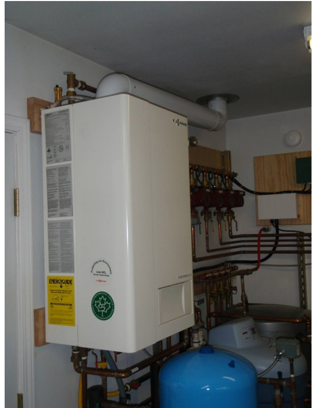
A Category 4, sealed combustion, condensing, power vented boiler.
