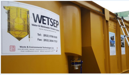
收集浮渣的出油盤 Oil Drain for Floating Scum
