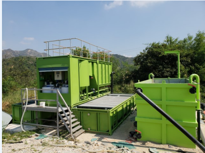
新界西堆填區 WENT Landfill
