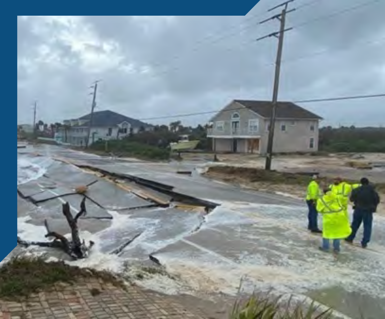
State Road A1A in Vilano Beach shortly after landfall of Hurricane Nicole.
