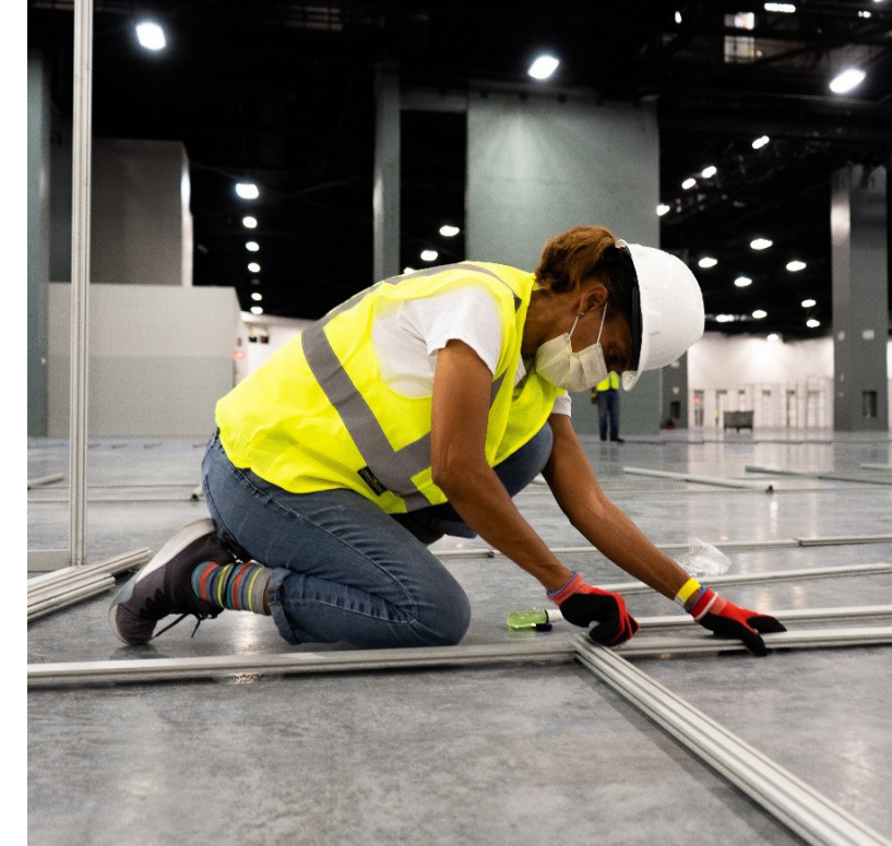
A construction worker takes measurements in advance of building a COVID Alternate Care Facility at the Miami Beach Convention Center in April. The U.S. Army Corps of Engineers Jacksonville District worked with state and local authorities to convert the 246,000-square-foot exhibition hall into a 450-bed field hospital. (Photo by Brigida Sanchez)
