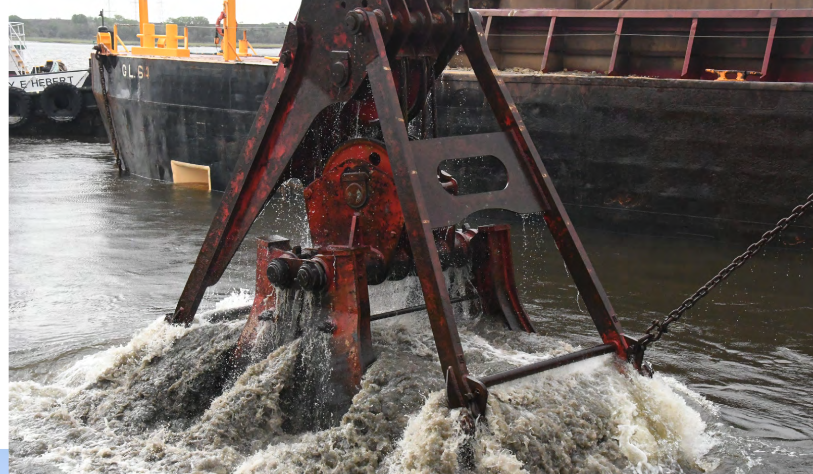
A clamshell dredger removes a batch from the river bed during a ribbon cutting ceremony that marked the completion of the Harbor Deepening Project at the Blount Island Marine Terminal Monday, May 23, 2022 at JaxPort in Jacksonville, FL. (USACE photo by Mark Rankin)
