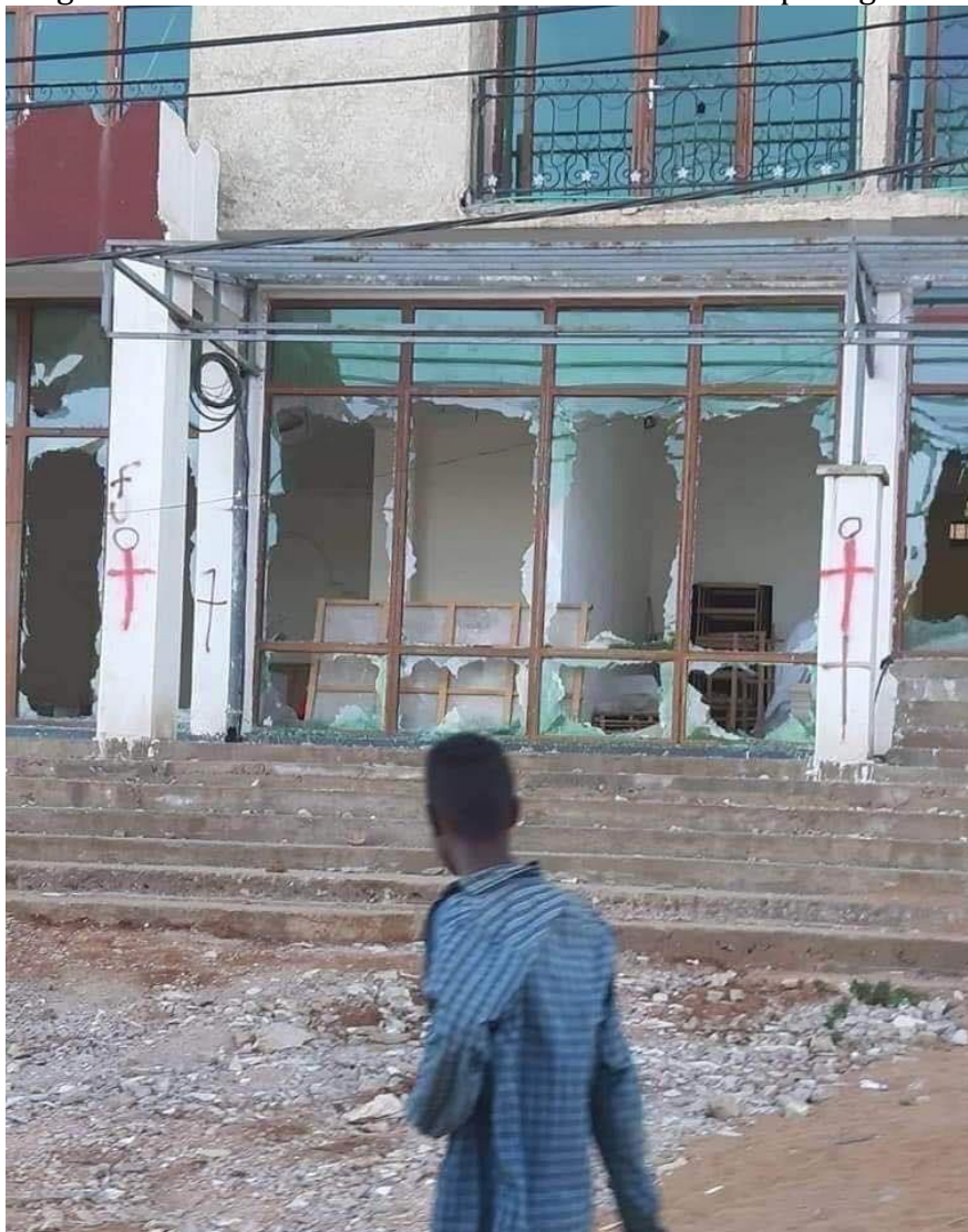
Damage incurred in Harar during violence in January 2020.
