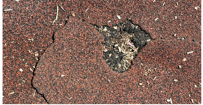
Traditional EPDM safety surface peeling away from the base layer
