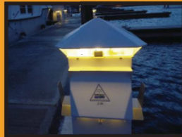
Protected KWH Counter
