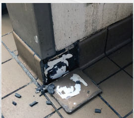
Base falling off wall
