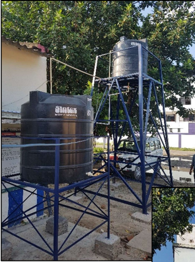
As and Fe removal in Bihar – India Gravity Asxban purifiers village- drinking water 2 m3/day
