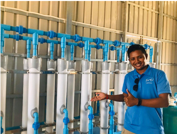
smartUF-Plant 15 m 3 /h Cambodia - pond
